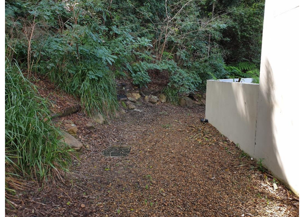
Photo B6: Inlet Pit at The Kilns
