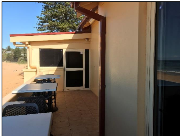
Figure 17. View of the open to sky terrace extended east from the Northern Wing. Note enclosed veranda extension behind the seating area. (Source: Heritage 21, 23.05.18)
