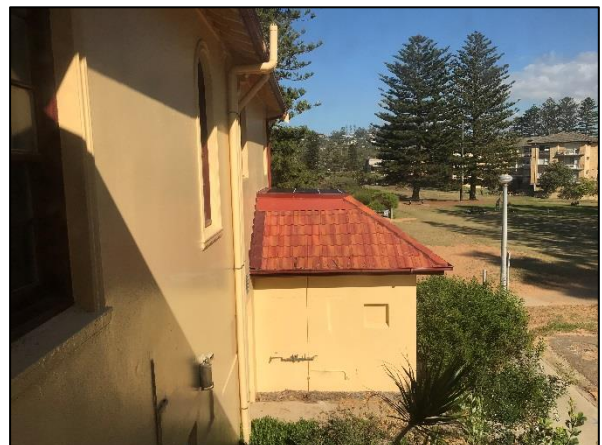
Figure 20. View of the Southern wing as seen from the office above the entry portico. (Source: Heritage 21, 23.05.18)
