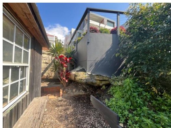
Photo 6: Rendered wall of the adjoining property to the north has built over undercut bedrock, on northern boundary in rear yard.
