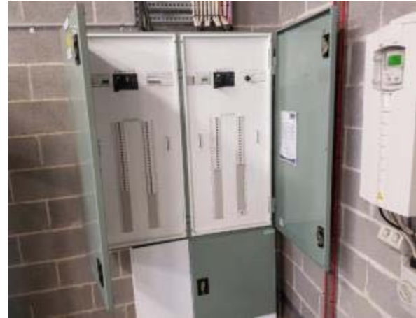
Space in DB board in Main switch room
