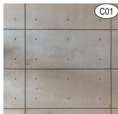
OFF FORM CONCRETE
