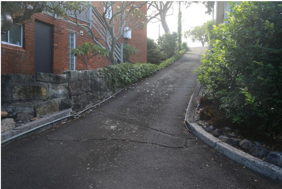
Figure 2.6 Access handle and driveway as viewed from the carport structure looking east towards Linkmead Avenue
