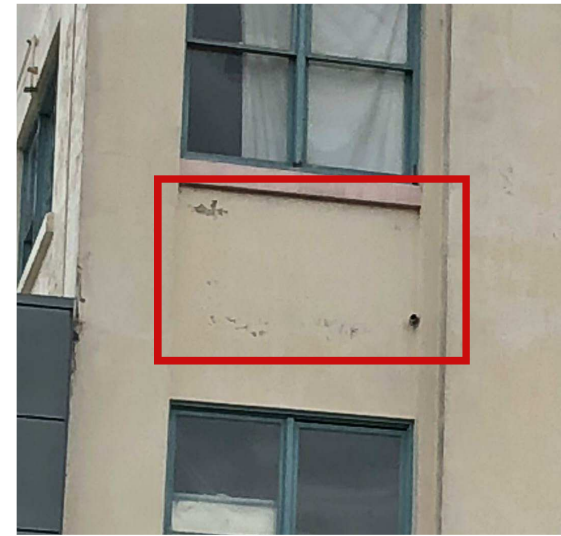
Investigate damp to building façade. Rectify cause and remove any salt laden render. Replace render to match original detail.
