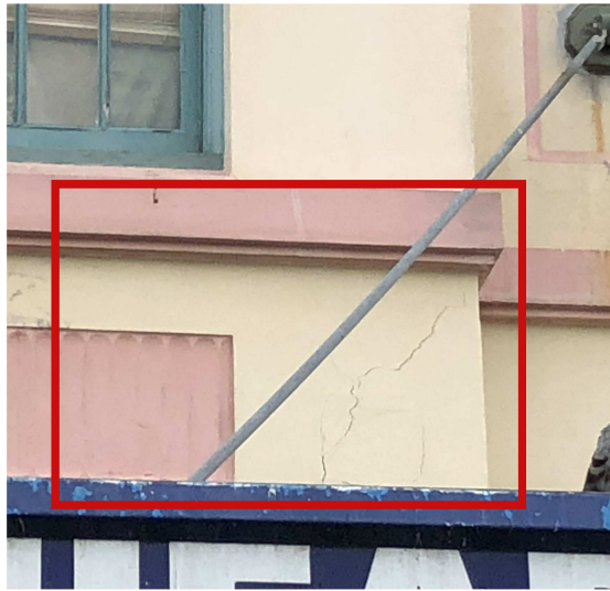
Open-up render and investigate extent of cracking. Rectify cracking to structural engineer and heritage architect's advice and reapply render to match original detail
