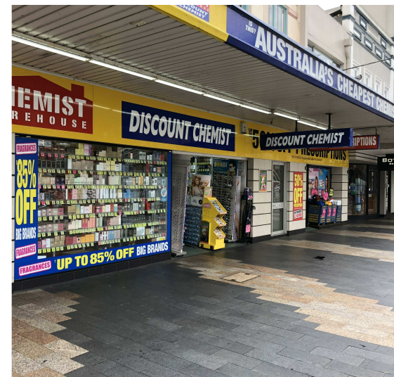
Retain and conserve existing shopfront awning. Open up and investigate possibility of any extant remnant original awning finishes. Rectify awning structure as required to structural engineer's advice. Reconstruct roof, fascia and soffit to match original detail if evident. (Allow for pressed metal soffit, marine ply fascia with timber trim, metal decking to roof and box gutter to building line)
