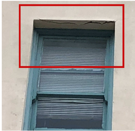
Open-up render and investigate extent of cracking. Rectify cracking to structural engineer and heritage architect's advice and reapply render to match original detail
