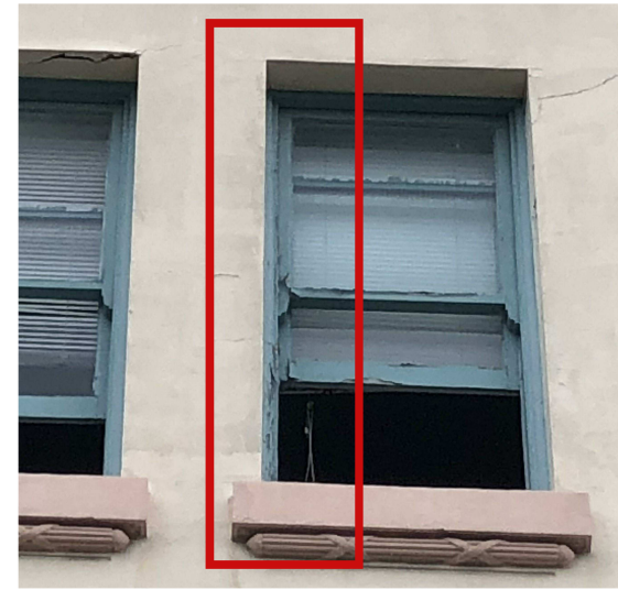
Open up render over all windows and investigate corrosion of lintels. Replace or rectify lintels to structural engineer and heritage architect's advice and reapply render to match original detail
