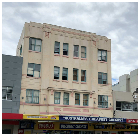
Allow to repaint entire façade and masonry returns to The Corso in heritage colour scheme based on paint scrape evidence performed on site once access to façade is provided. Paint shall be Dulux Acratex Acraseal or similar to heritage architect's approval.
