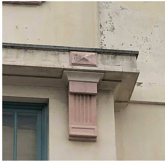
Open up and investigate cracking to pediment. Rectify cracking to structural engineer and heritage architect's advice and reinstate rendered detail to match original.
