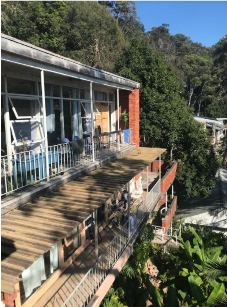
Photo 1: Existing balcony areas from No. 10 Taminga from No.11 Taminga rear balcony areas.
