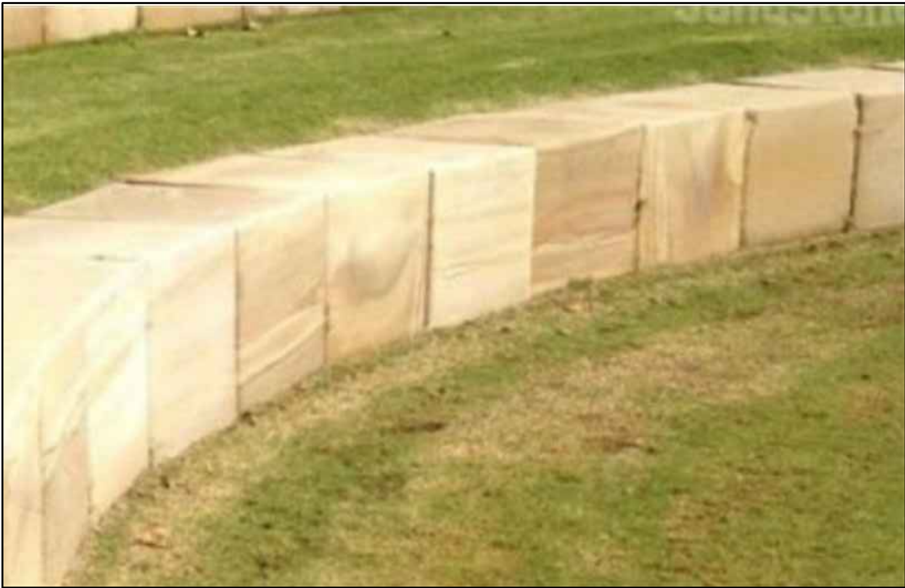
SANDSTONE LOGS RETAINING WALL
