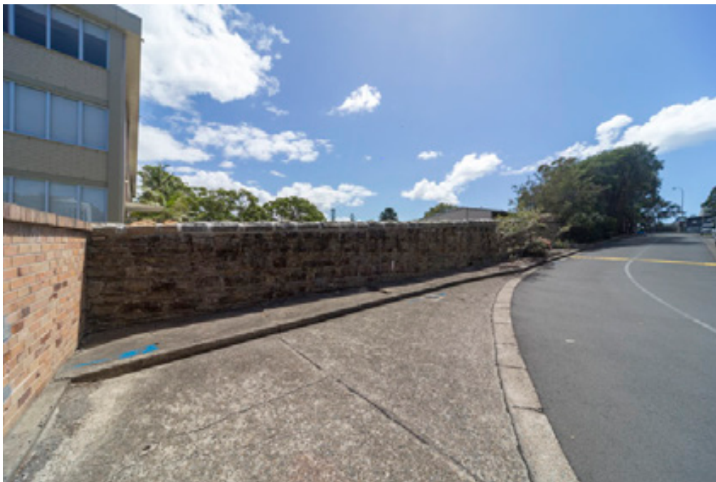
Figure 38: The southern end of the western boundary wall of the core hospital site
