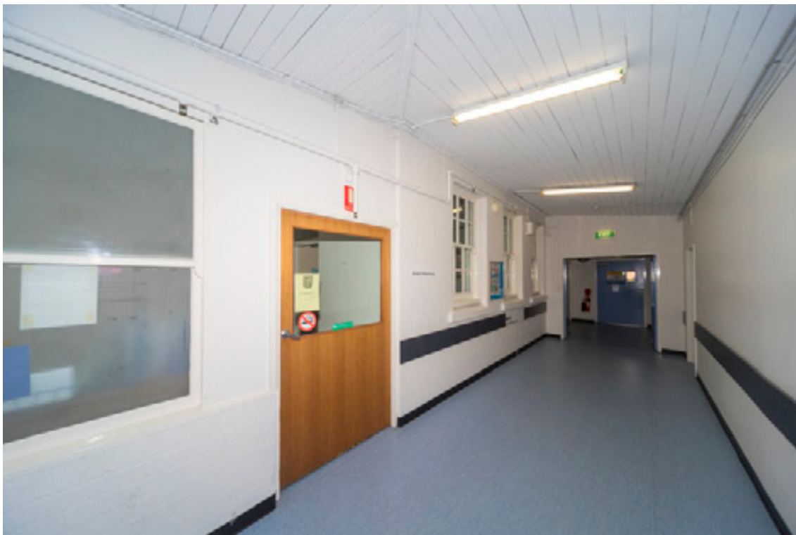
Figure 57: View of the northern wall of Bulding 15, looking west with original windows (centre) and original timber verandah ceiling
