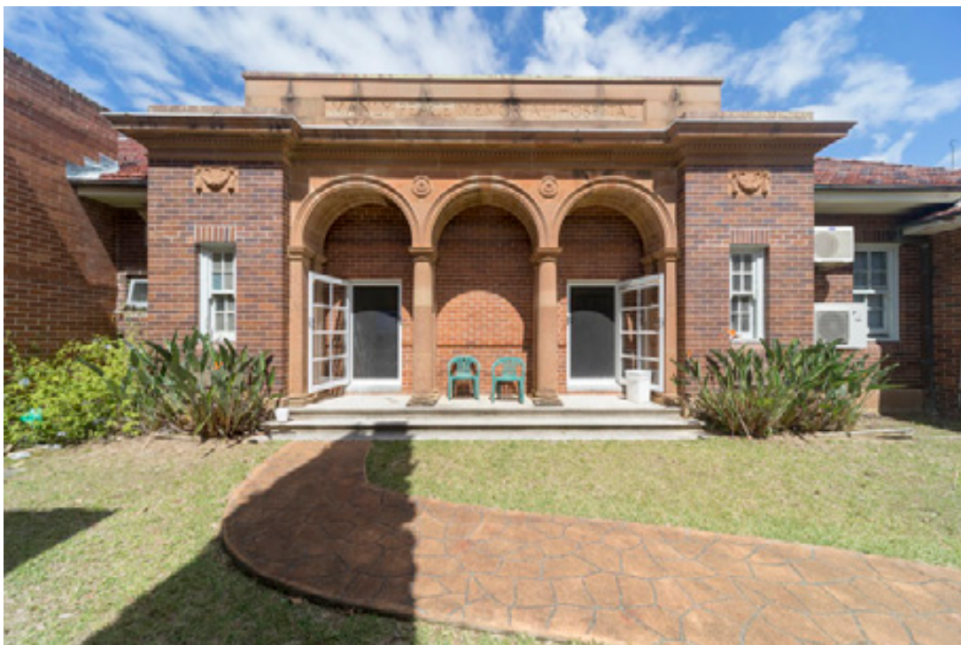
Figure 101: The remnant façade of Building 1. This is virtually all that remains of the north elevation of the original 1928 Building 1. The wall behind the sandstone arches was constructed in 1992.
