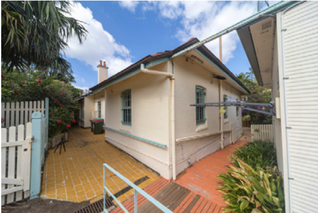
Figure 80: The west and (at left) part of the north elevation of Parkhill cottage. Note metal shed addition at right, to the west of Parkhill house.
