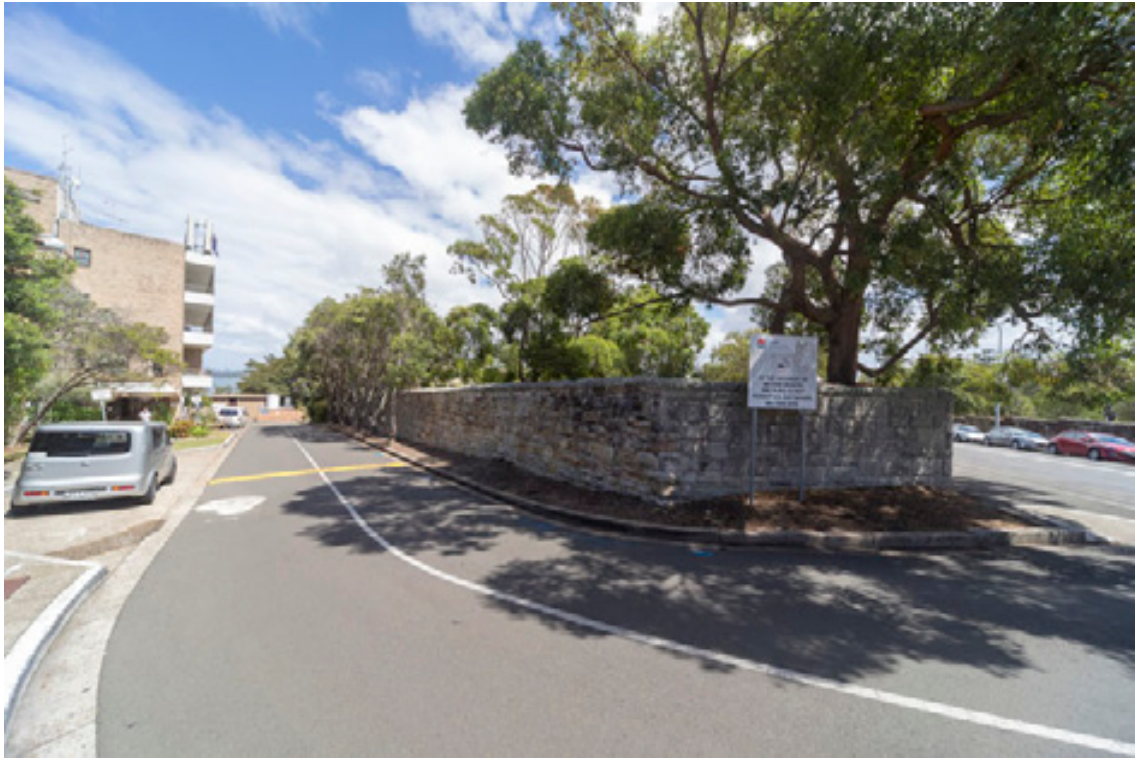
Figure 37: The northern end of the western boundary wall of the core hospital site.
