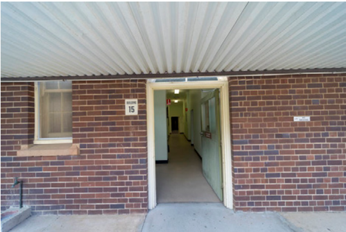
Figure 53: South elevation ground floor entry into Building 15. Note original window at left with sandstone sill.
