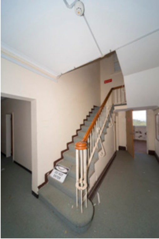
Figure 69: (Left) Original staircase with steel balustrading and timber handrail to Building 22 Level 1 interior
