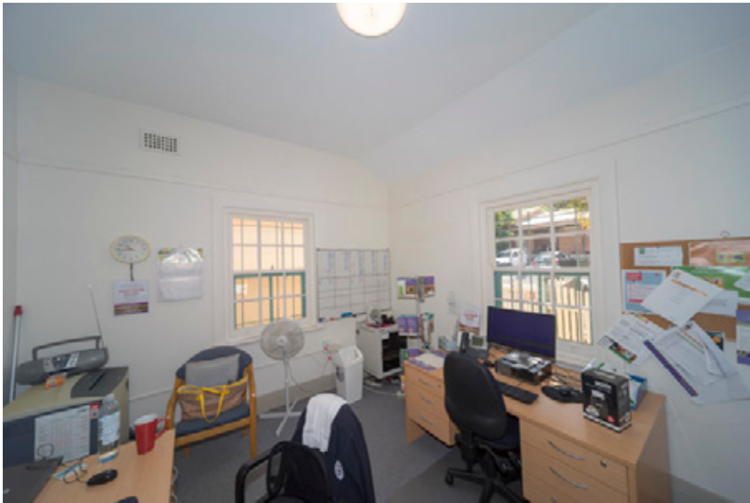
Figure 88: Interior view of office to south-western corner of Parkhill cottage showing original windows, picture rails, skirting boards
