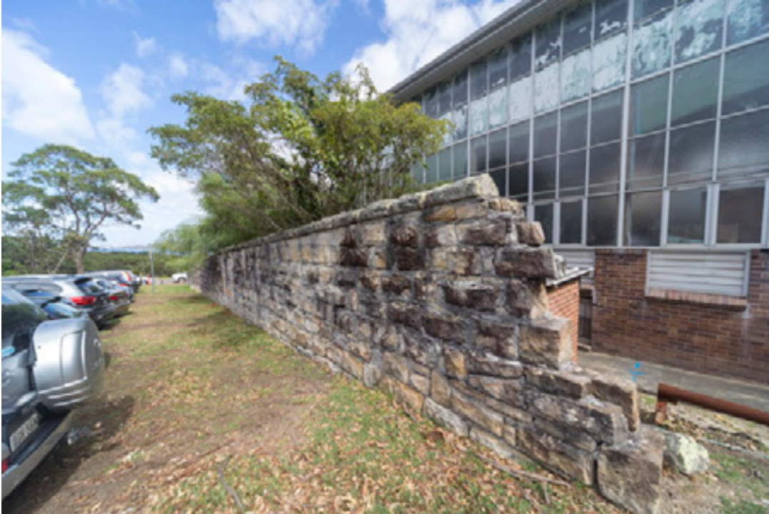
Figure 32: The northern end of the Eastern boundary wall of the original hospital site, from the north-east, looking south showing where the wall has been demolished adjacent to Building 13
