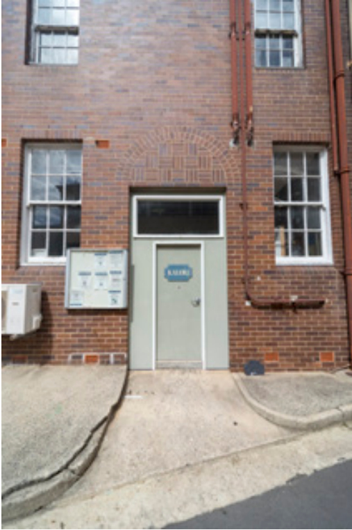
Figure 65: (Left) Detail of doorway with later doors to north elevation of Kalori, Building 22, noting original windows, brickwork including elaborate brickwork over doorway.
