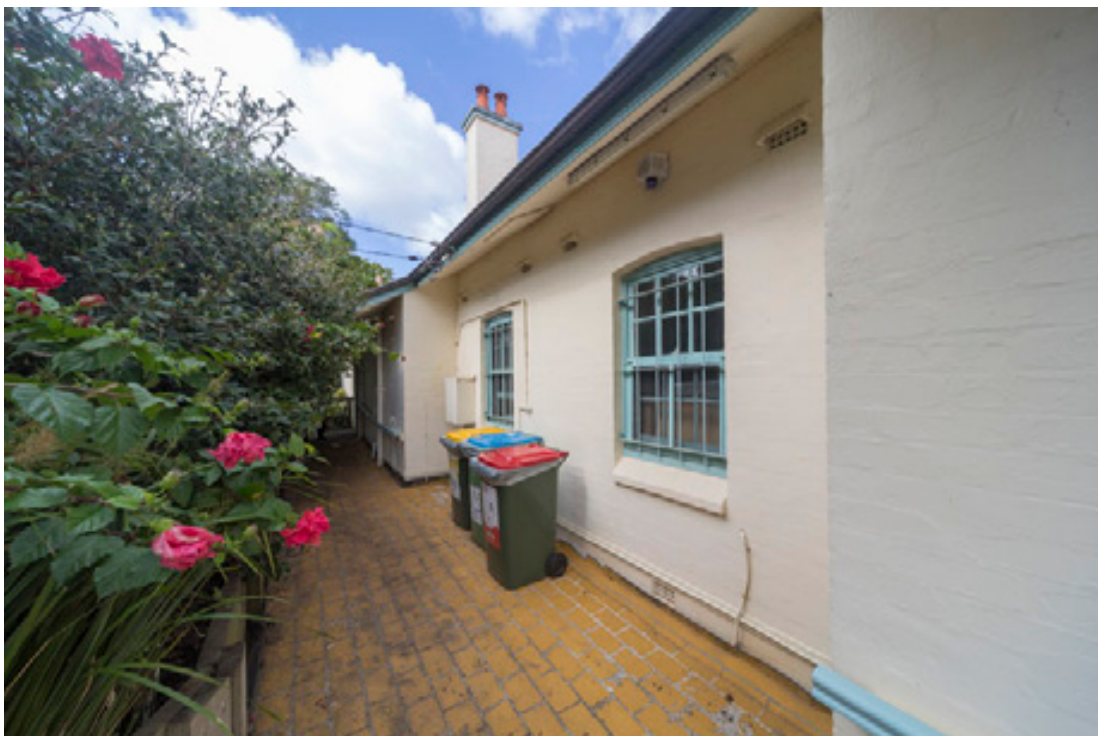
Figure 77: Western end of the north elevation of Parkhill cottage showing original timber framed multi-paned windows.
