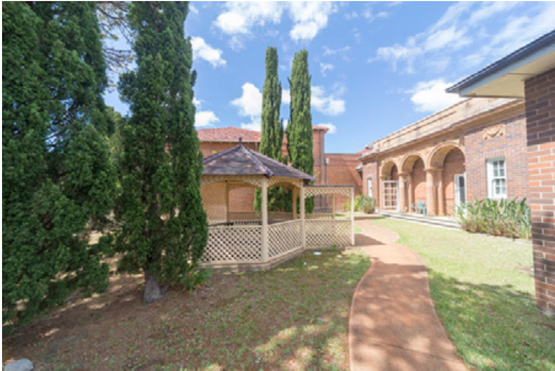
Figure 100: View towards the remnant façade of the 1928 Building 1 (right) with the west elevation of Building 30 beyond and a recent summer house (centre)
