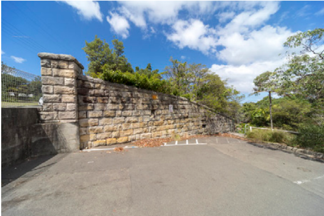
Figure 35: North end of the eastern boundary wall of the core hospital site, adjacent to car park P6. This is a view of the western side the wall.
