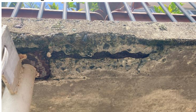
Image of balcony showing concrete cancer
