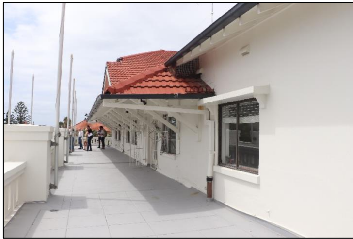
Figure 21: The hipped roof to the centre and eastern section of the elevation.
