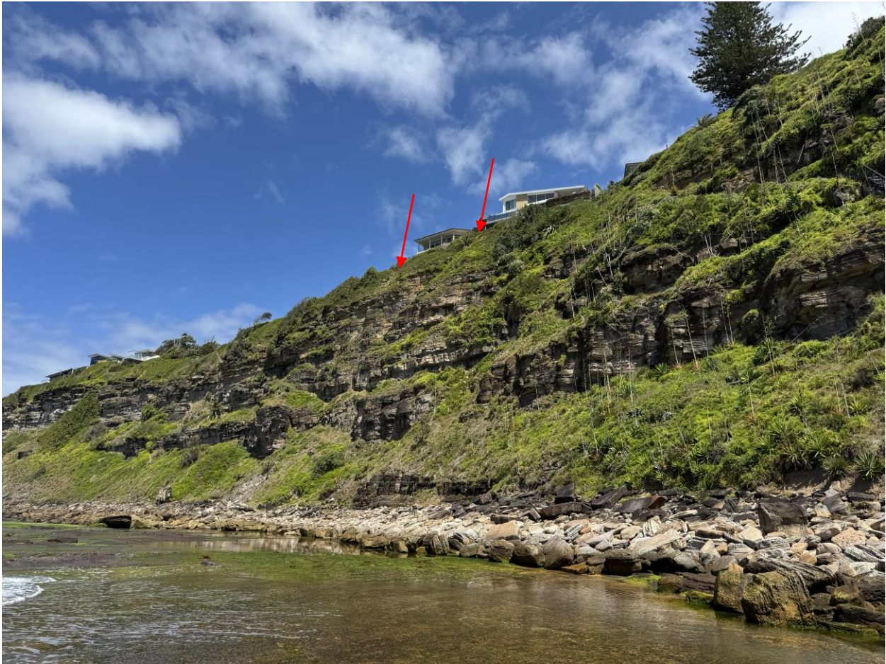
Figure 3: View of cliff face at site (extent at top of cliff approximately between arrows) on 3 October 2024, facing SSW
