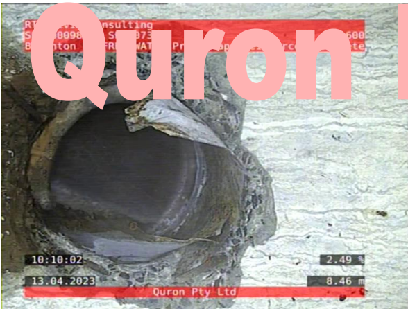
3, 00:02:47, 8.46 Connection, poor workmanship, connection appears to be open, height: 100mm at 11 o'clock
