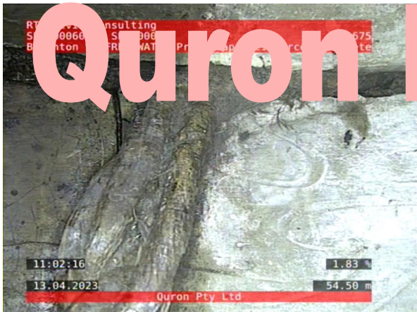
3, 00:19:16, 54.50 Tap roots--a small number of major roots (10mm or greater) without a significant mass of fine root, at joint, Obstruction: <5% at 4 o'clock
