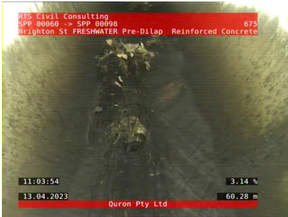
5, 00:20:25, 60.28 Fine roots--a relatively small number of flexible minor roots, Obstruction: 5-20% from 5 o'clock to 7 o'clock, Start #
