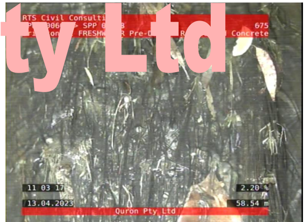
4, 00:20:04, 58.54 A mass of mostly fine roots, which has developed into an interwoven clump, Obstruction: 5-20% from 4 o'clock to 8 o'clock
