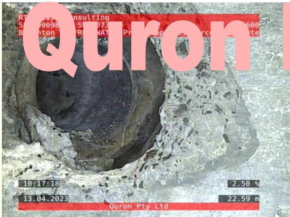
7, 00:07:02, 22.59 Connection, poor workmanship, connection appears to be open, height: 100mm at 10 o'clock
