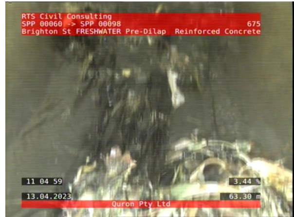
6, 00:21:14, 63.30 A mass of mostly fine roots, which has developed into an interwoven clump, at joint, Obstruction: 5-20% from 4 o'clock to 8 o'clock
