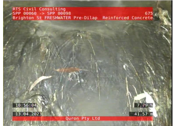
2, 00:15:41, 41.57 A mass of mostly fine roots, which has developed into an interwoven clump, at joint, Obstruction: 21-50% from 4 o'clock to 8 o'clock
