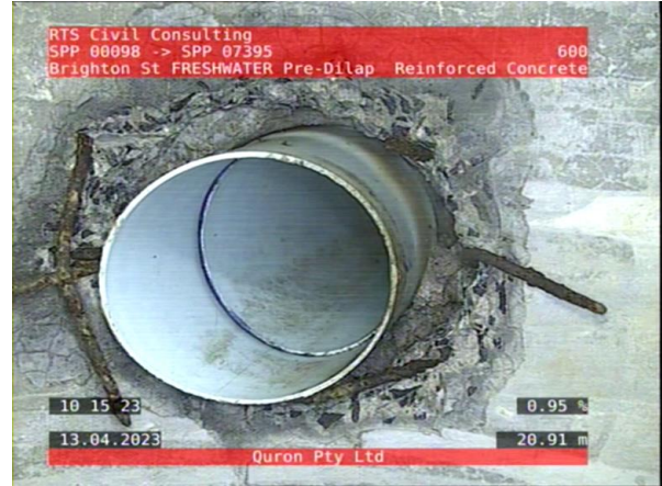
6, 00:06:14, 20.91 Reinforcement is exposed and corroded at 1 o'clock
