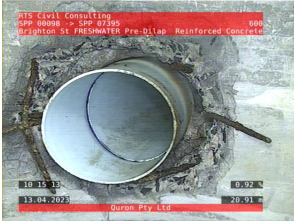
5, 00:06:10, 20.91 Connection, poor workmanship, connection appears to be open, height: 100mm at 1 o'clock
