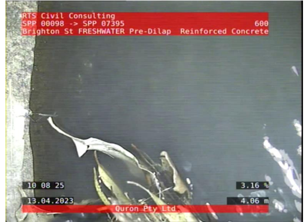
2, 00:01:26, 4.06 Tap roots--a small number of major roots (10mm or greater) without a significant mass of fine root, at joint, Obstruction: 5-20% from 6 o'clock to 8 o'clock, Finish #
