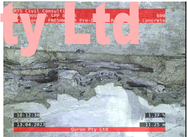
4, 00:03:49, 11.25 Reinforcement is exposed and corroded, at joint from 11 o'clock to 1 o'clock
