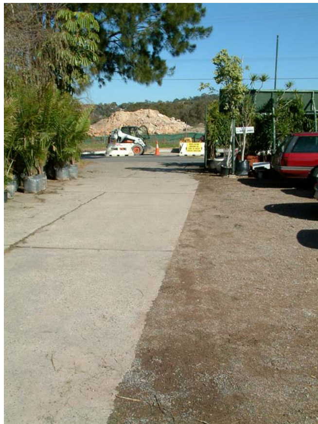
Plate 6: Example of the graded driveways/through affairs and levelled working areas within the study area.
