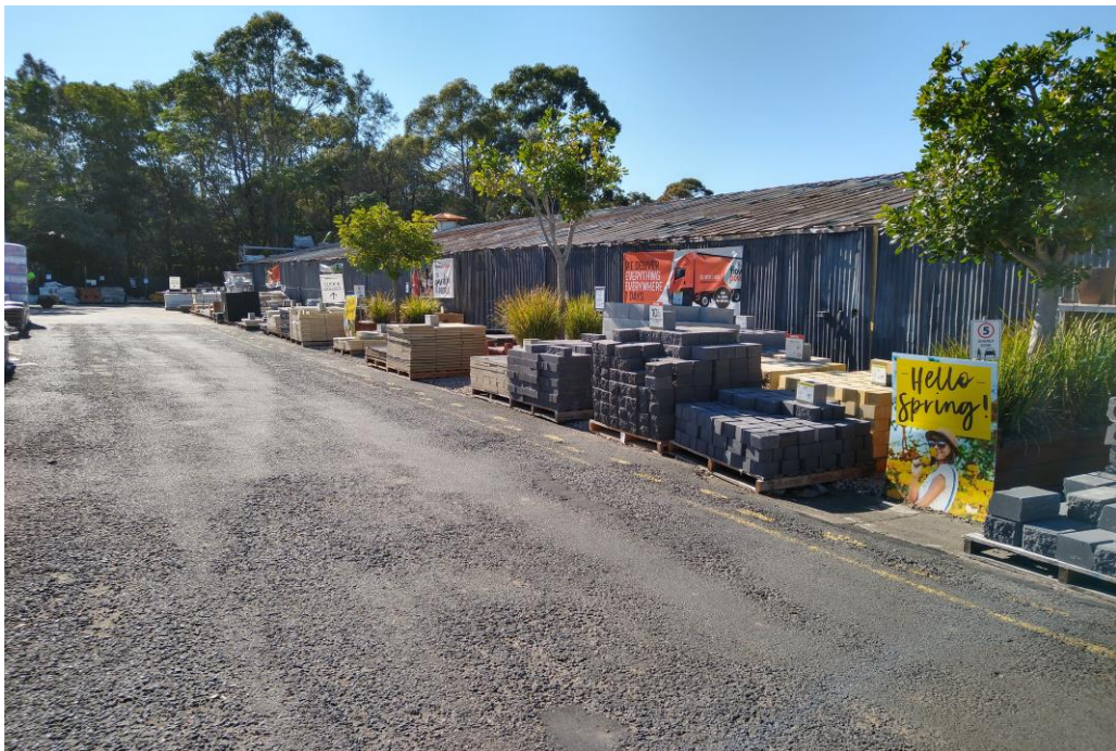
Photo 10 – Building material placed along the site road through the middle of the site (beside plant nursery)
