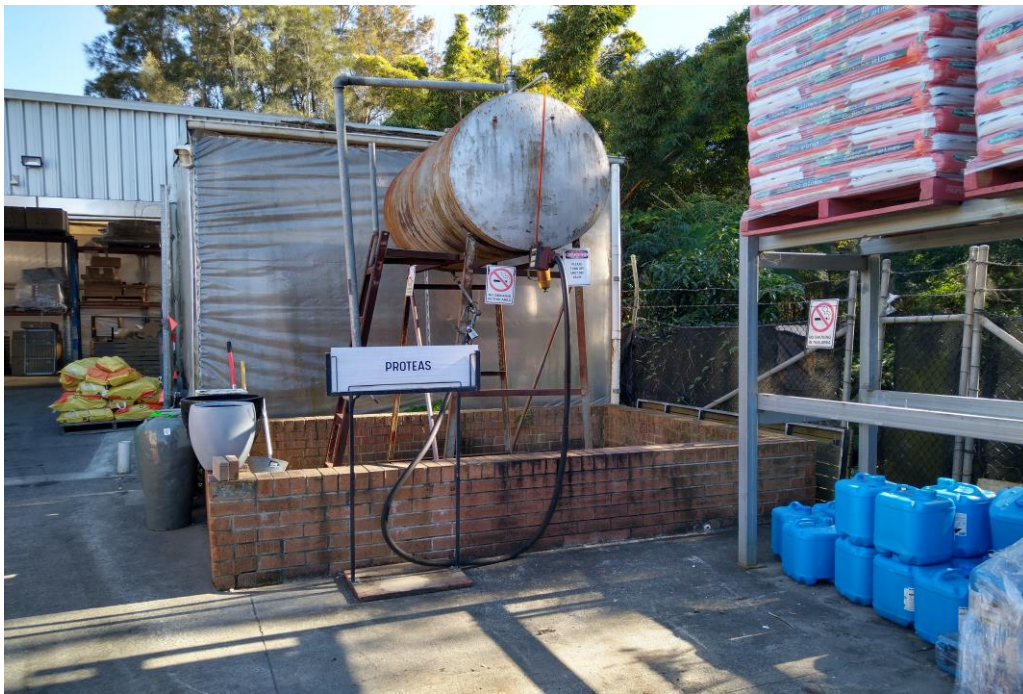
Photo 12 – Above-ground diesel tank in northern portion of site
