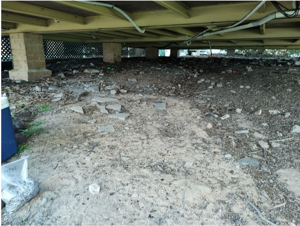
Photo 5: NNPS – Suspected asbestos-containing fibre cement material observed in northern part of investigation area.
