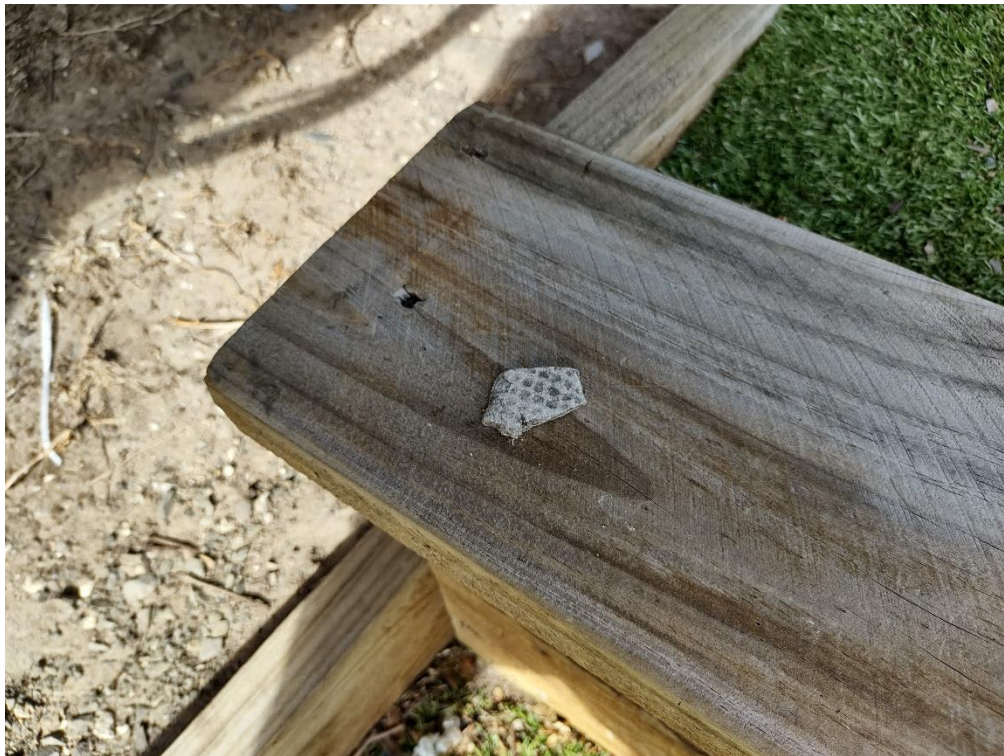
Photo 6: NNPS – Asbestos-containing material (A02) sampled in northern part of investigation area.
