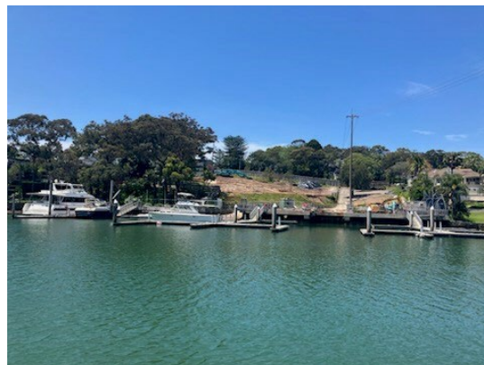
Photograph 4: View of corroded steel sheet piling beneath the concrete capping including the small boats ramp and boat lift section
