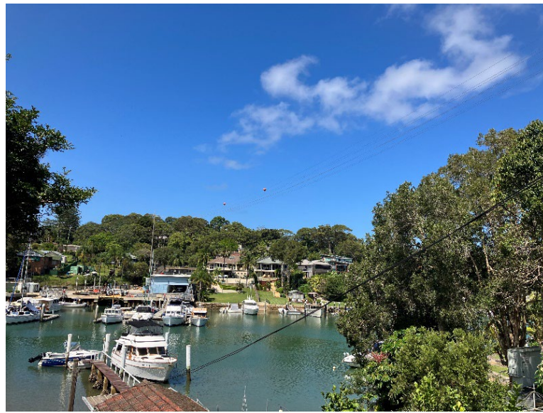
Photograph 2: High voltage cables (with red balls) over Winji Jimi Bay and suspended above Lot 5
