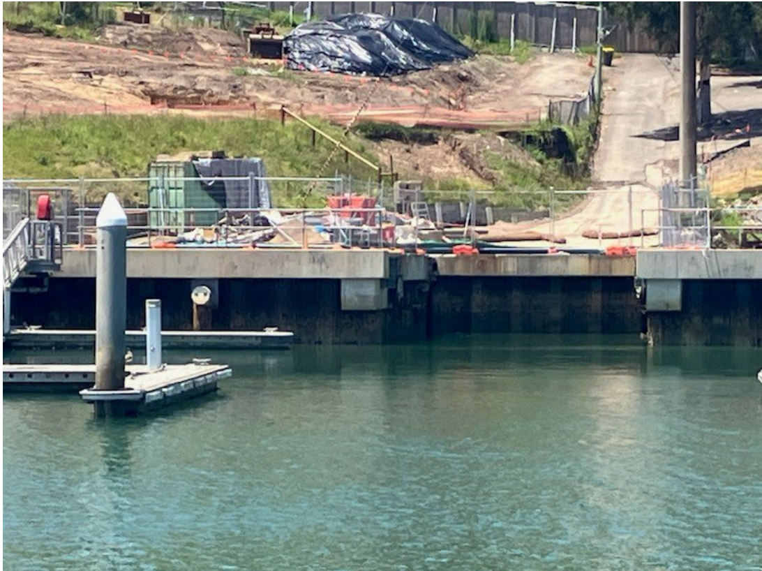
Photograph 5 Close-up view of existing seawall showing deterioration including holes in the sheet piling and the existing boat lift section
