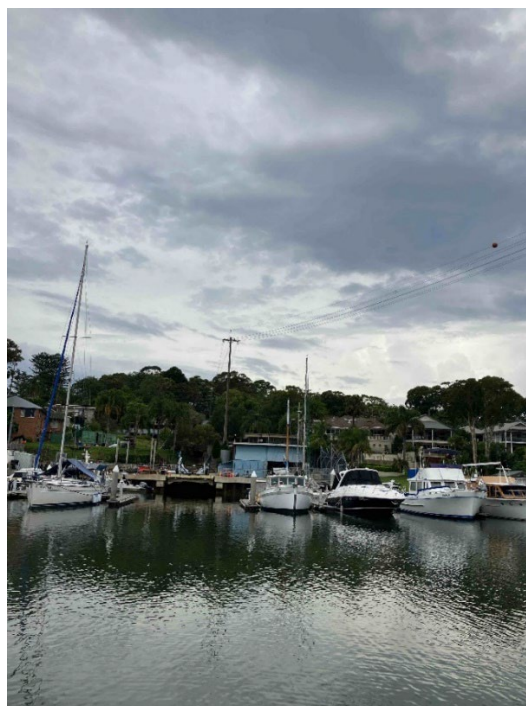
Photograph 3: High voltage cables over Winji Jimi Bay and over the proposed Lot 5
