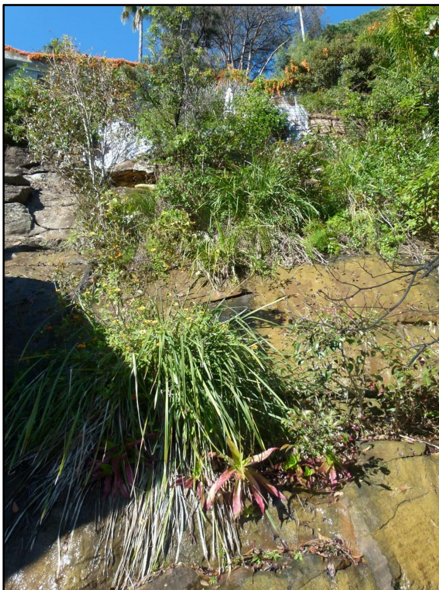
ROCK FACE AT REAR OF 17 FLORIDA ROAD SHOWING ROCK PILE AT TOP OF THE CLIFF
