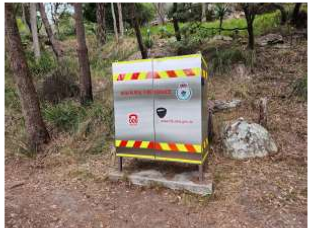
Existing Hose Post (RFS)
