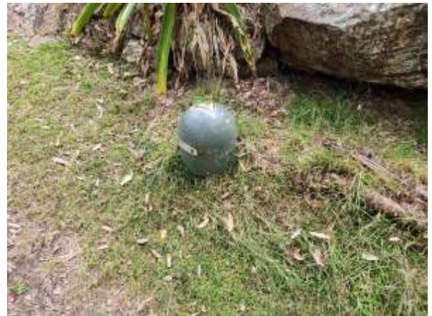
Underground electrical supply
