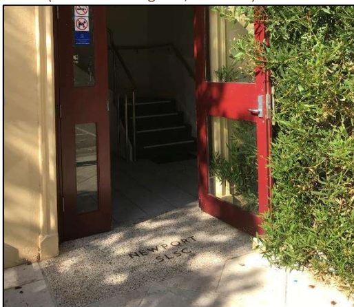
Figure 54. Detail of main entrance, featuring entry threshold with metal letters. (Source: Heritage 21, 23.05.18)
