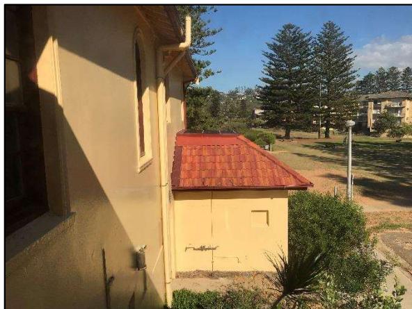
Figure 102. View of the Southern wing as seen from the office above the entry portico. (Source: Heritage 21, 23.05.18)
