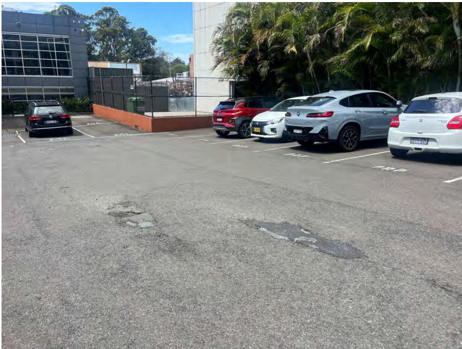
Photograph 2: Rear of 1753 Pittwater Road); pavement showing cracks and stains
