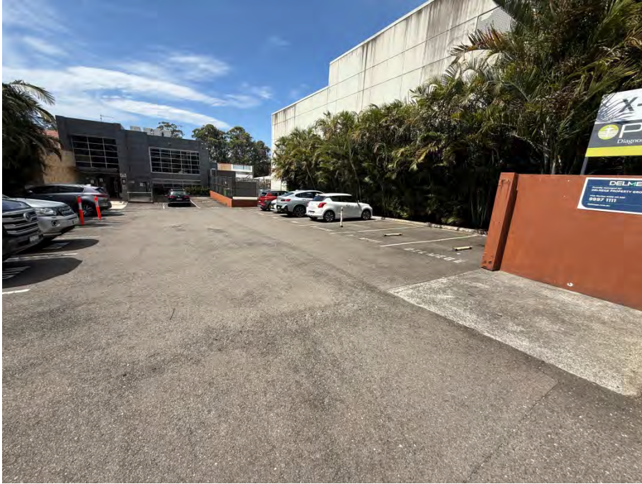
Photograph 1: Rear of 1753 Pittwater Road; pavement showing cracks and stains
