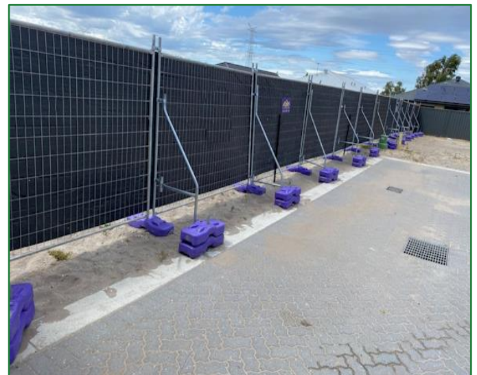
Photo 4. Temporary Environment Protection Fencing with Bracing & Shade Cloth (Suitable for Windy Conditions)
