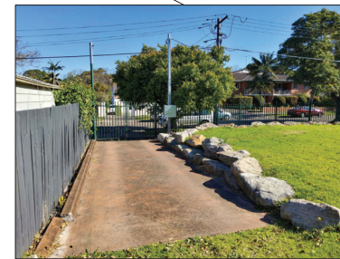
EXISTING HARDSTAND ALONG NEIGHBOURING PROPERTY TO BE DEMOLISHED AND GATE TO BE RELOCATED TO THE NEW EGRESS
