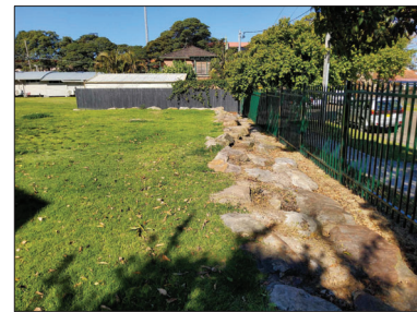
EXISTING ROCK RETAINING WALL ALONG SOUTHERN BOUNDARY TO BE REMOVED. FENCE TO BE RETAINED
