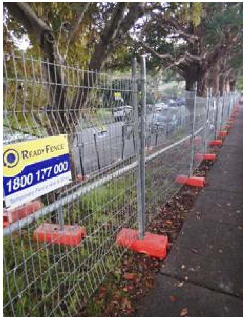
Example image of acceptable tree protection fencing measures to be applied. (1.8m high rigid metal fencing with appropriate lateral bracing)
