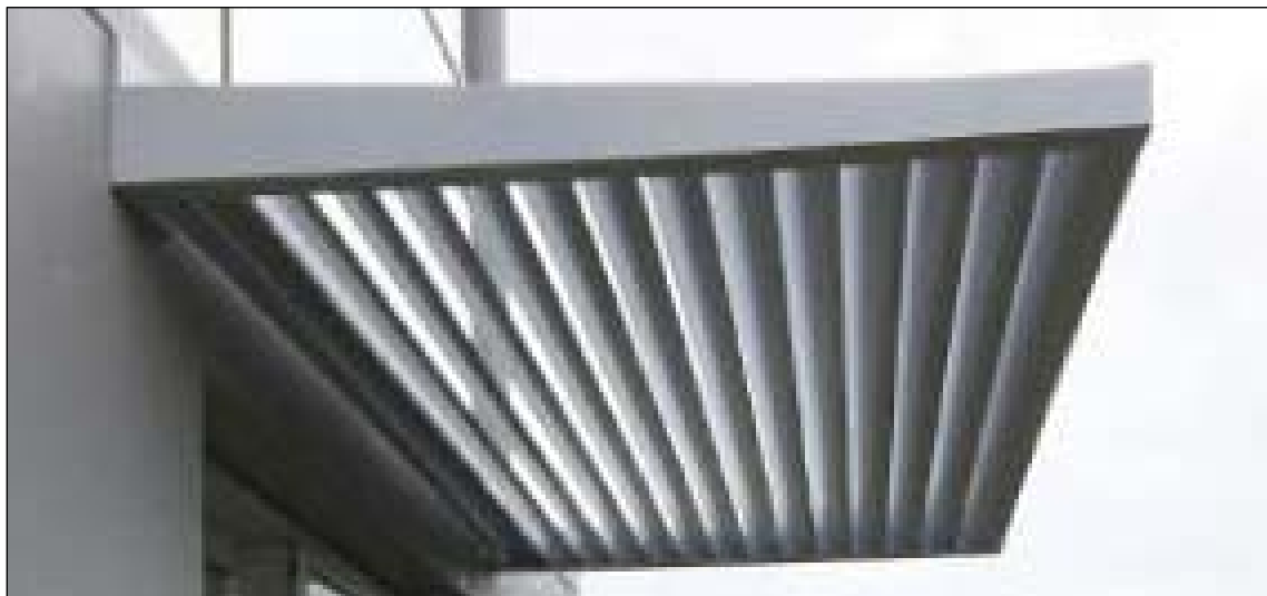
Window Awnings Aluminium Louvre Awnings above windows for Sun Control
