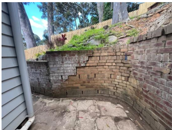
Photo 5: Damaged return (eastern side) of the brick wall at the dwelling rear
