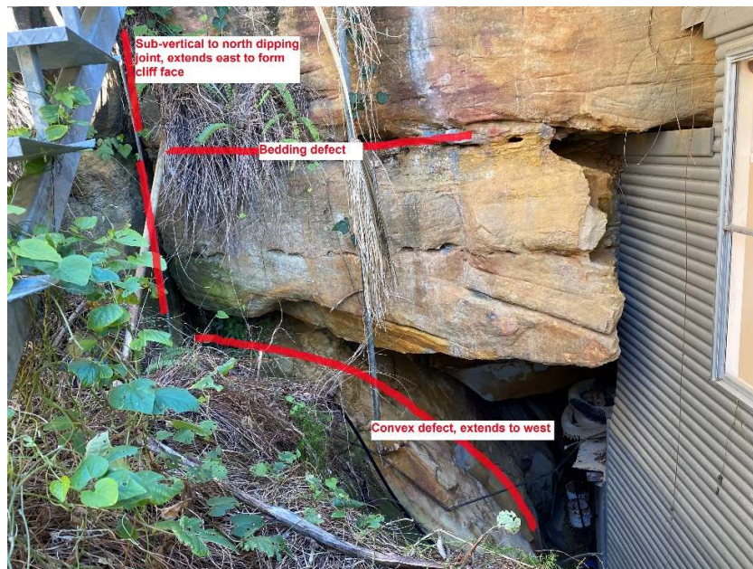
Photograph 9: Defects within bedrock and overhang/undercutting at south-west corner of existing house.
