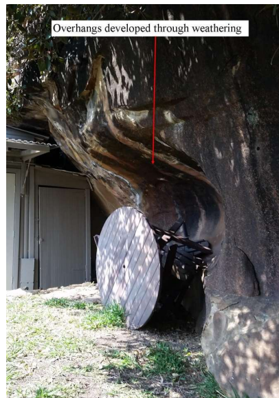
Photograph 8: Overhang/undercutting within the site.
