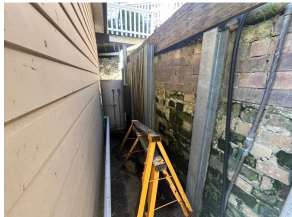
Photo 4: Brick wall at the rear of dwelling reinforced with steel beams. Showing signs of significant bulging
