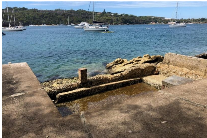
Figure 1: 16 Addison Road Manly – the dilapidated harbour swimming pool & concrete paving
