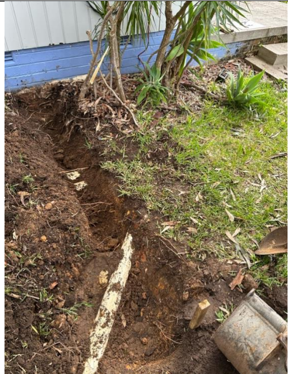
Figure 8 shows root investigations carried out by the client
