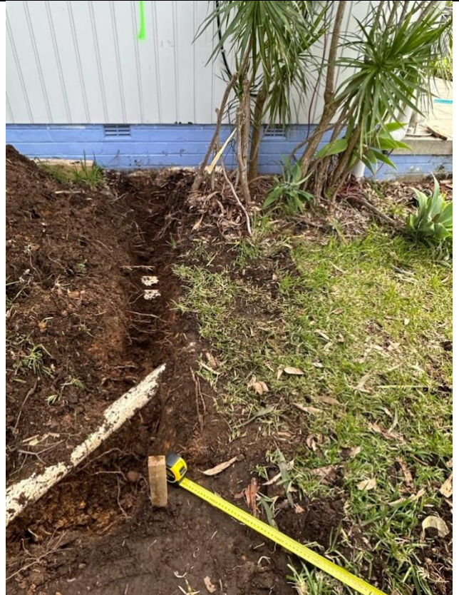
Figure 6 a trench for the proposed footings, no large roots can be seen
