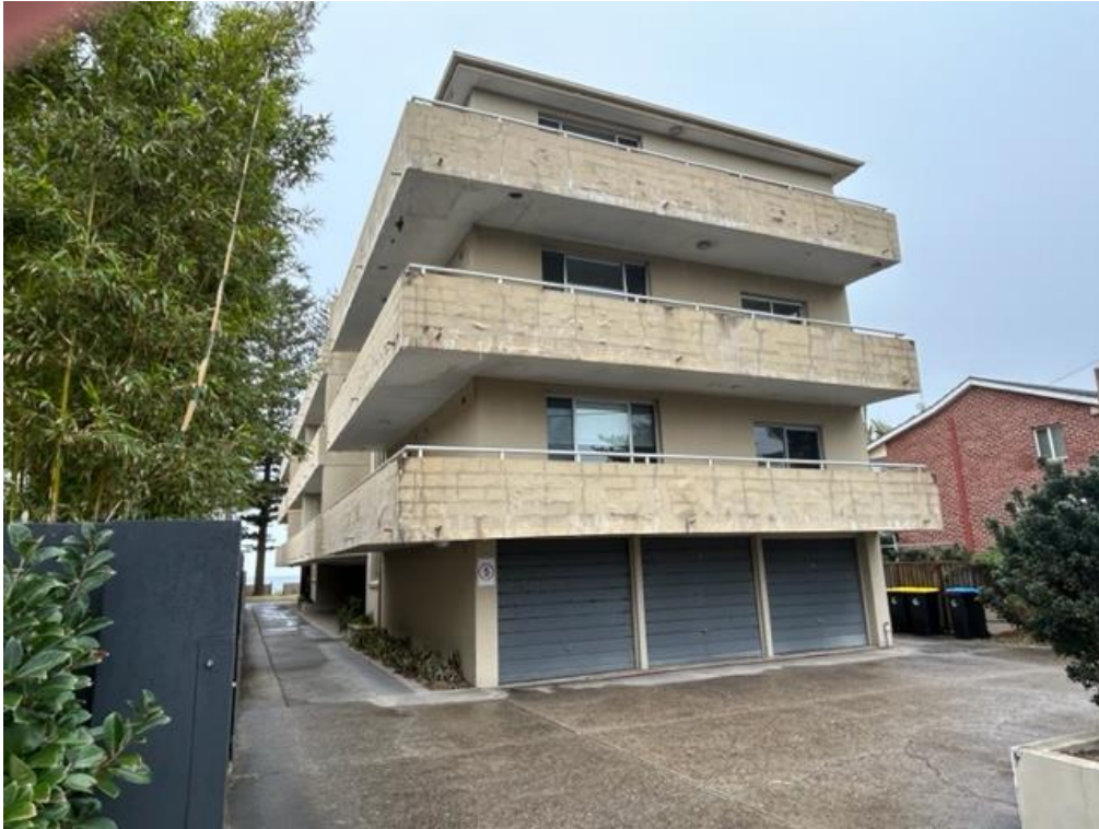
Photograph of the site, Northern Façade – 157 Ocean Street, Narrabeen Note deteriorating balconies, dated garage doors and driveway damage
