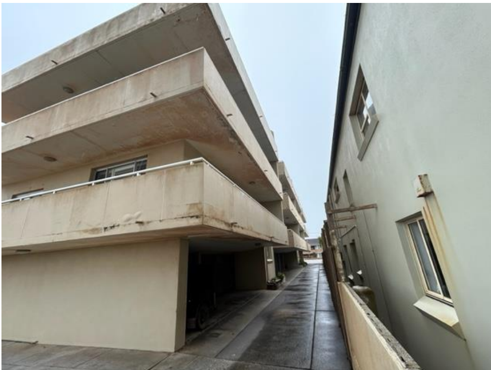
Photograph of the site, Northern Façade – 157 Ocean Street, Narrabeen Note concrete cancer, Balcony damage
