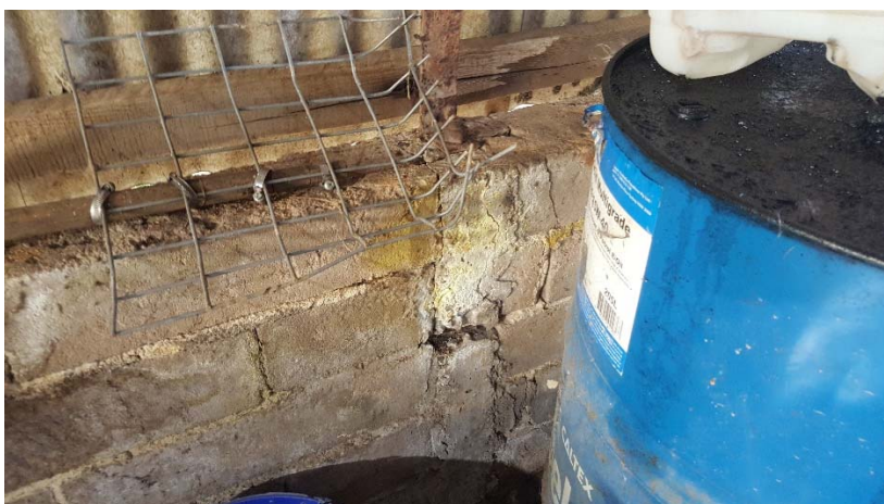
Frame 2 & 3 – Block retaining wall forming part of existing metal shed found to be structurally inadequate.
