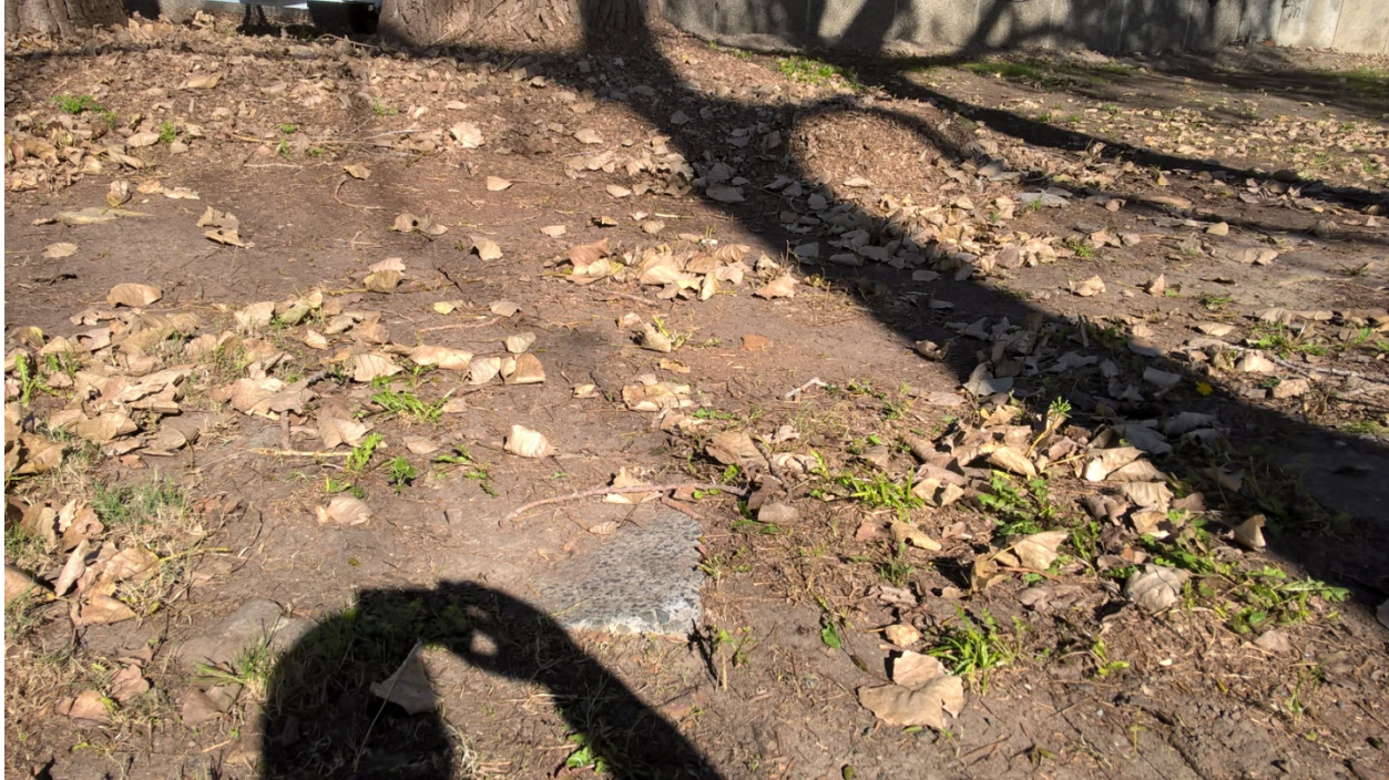
Photographic Plate 10: Possible footing of former fence post or small shed structure in southwestern corner of the subject site, southern perspective
