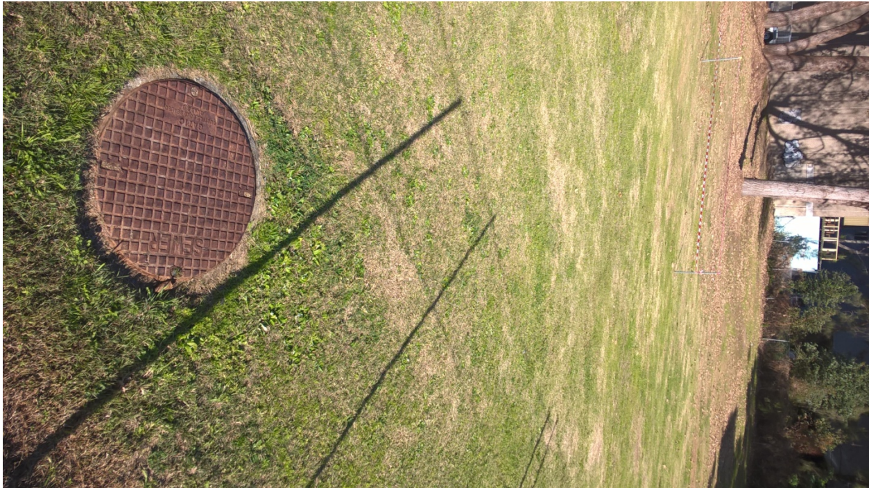
Photographic Plate 7: Sewer main access gatic located approximately 55 metres west of the Lot 201 / 202 DP 1019363 property boundary, southern perspective from Jubilee Avenue fenceline
