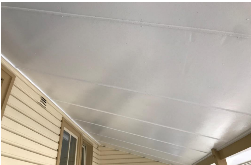
Photograph 4: B00J, exterior, movement (balcony), ceiling, fibre cement sheeting, asbestos detected by analysis.
