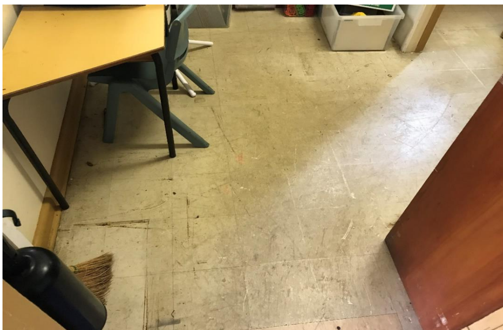
Photograph 8: B00P, R0003 - Storeroom, floor, vinyl tiles, asbestos (assumed).
