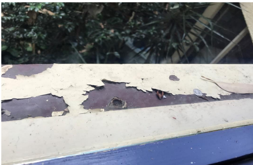
Photograph 3: B00A, exterior, throughout, walls, white paint, positive for lead.
