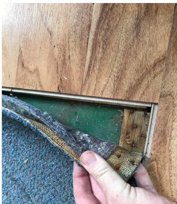
Photograph 6: B00H, R0005 - Staff Room, floor, vinyl tiles (green), asbestos detected by analysis.
