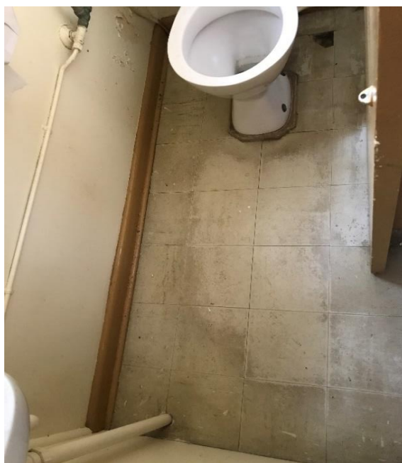
Photograph 6: B00P, R0001 - Staff Toilet, floor, vinyl tiles, asbestos detected by analysis.
