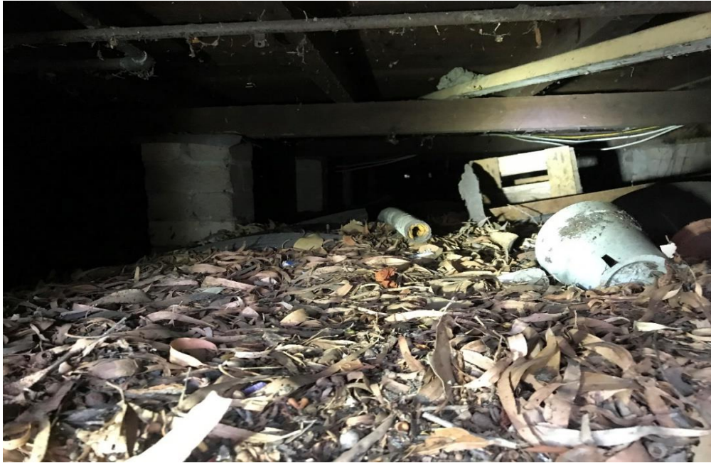
Photograph 1: B00P, exterior, subfloor, packing to piers beneath metal ant cap, fibre cement fragments, asbestos (assumed).
