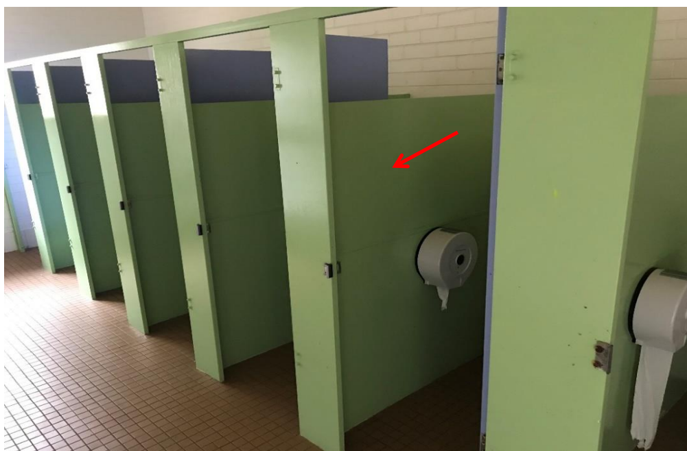
Photograph 4: B00R, R0009 - Girls Toilet , partition walls, compressed fibre cement, asbestos detected by analysis.
