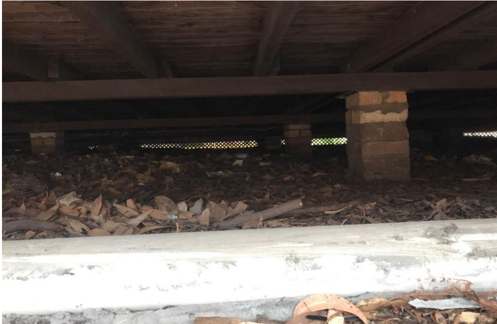
Photograph 1: B00H, exterior, subfloor, underfloor voids, packing materials, fibre cement fragments, asbestos detected by analysis.
