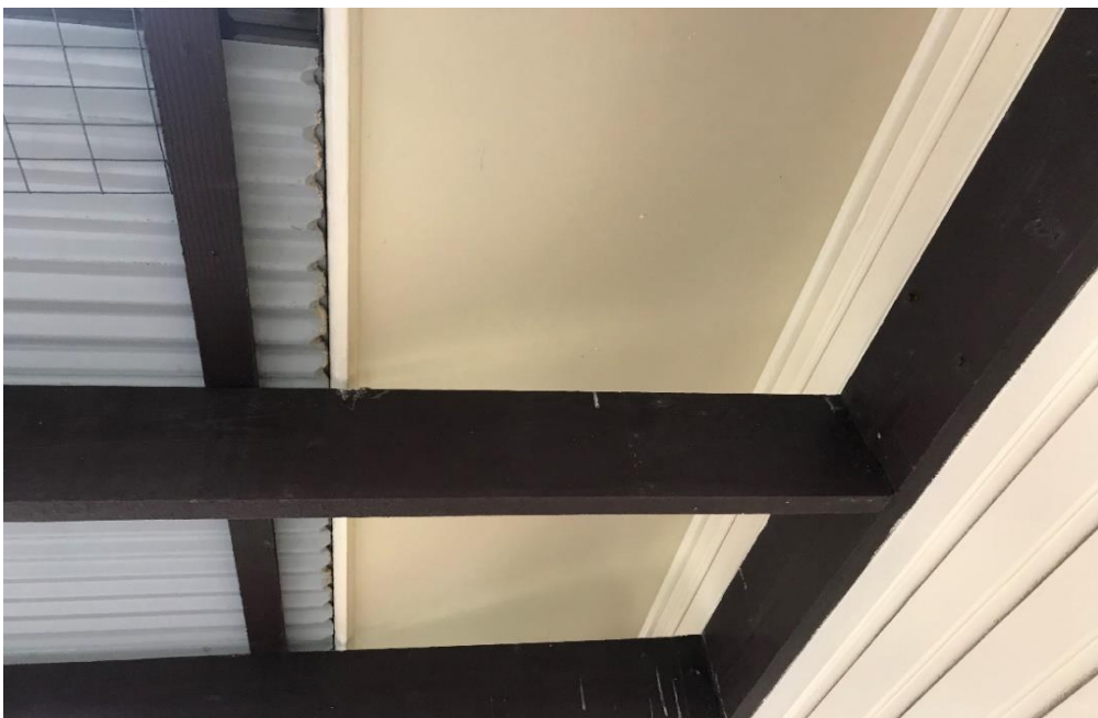
Photograph 4: B00P, R0010 - Movement (balcony), ceiling/eave, fibre cement sheeting, asbestos detected by analysis.
