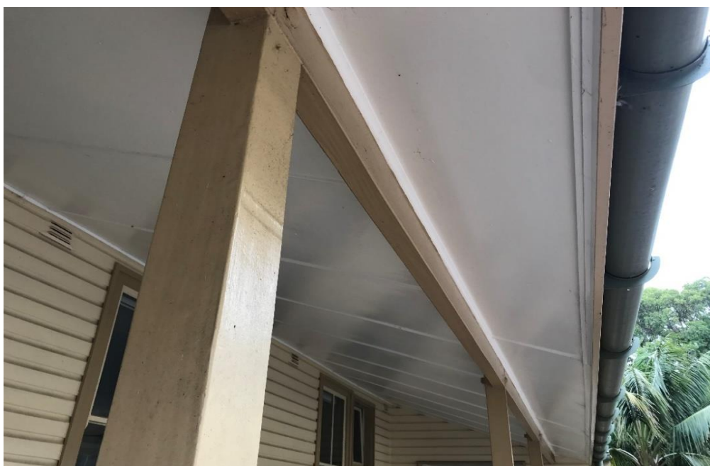
Photograph 2: B00J, exterior, eaves, fibre cement sheeting, asbestos detected by analysis.
