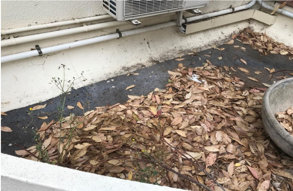
Photograph 1: B00B, exterior, north eastern garden beds, lining to garden bed , bituminous membrane, asbestos (assumed).
