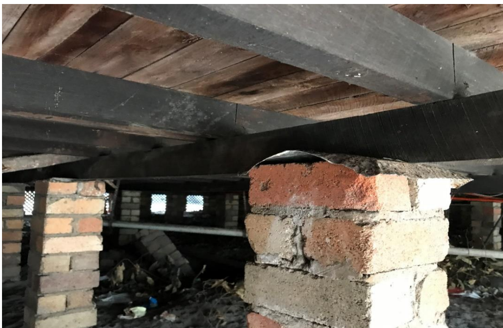
Photograph 1: B00J, exterior, subfloor, on brick piers between stilts and ant cap, fibre cement fragments, asbestos detected by analysis.
