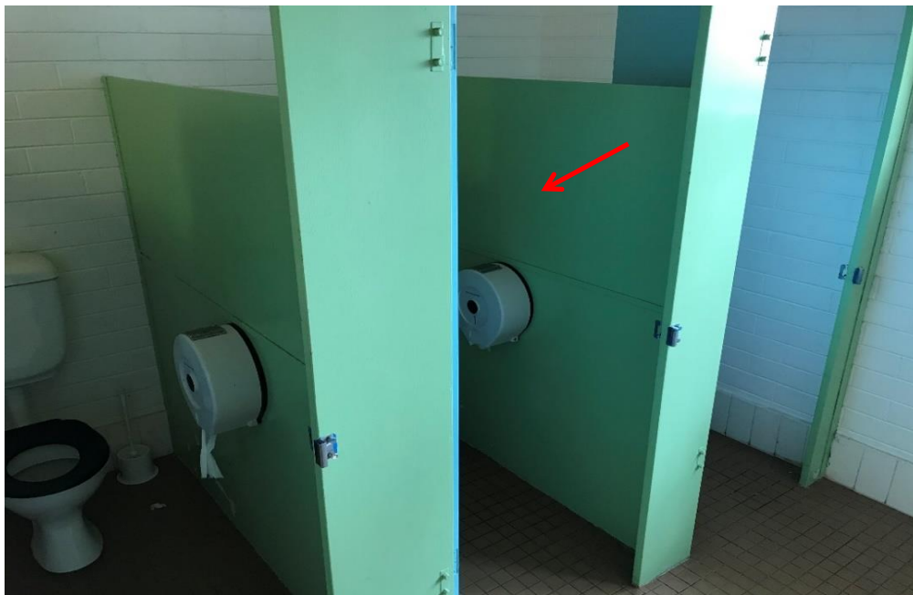
Photograph 2: B00R, R0010 - Boys Toilet, partition walls, compressed fibre cement, asbestos detected by analysis.
