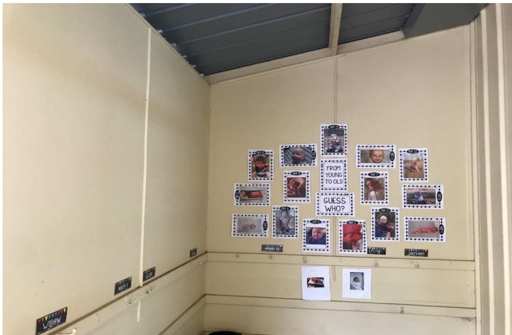
Photograph 2: B00N, R0003 - Movement (Balcony), wall linings to east and west walls , fibre cement sheet, asbestos detected by analysis.
