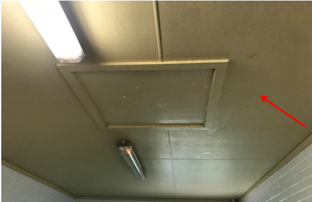
Photograph 1: B00R, R0010 - Boys Toilet, ceiling, fibre cement sheet, asbestos detected by analysis.
