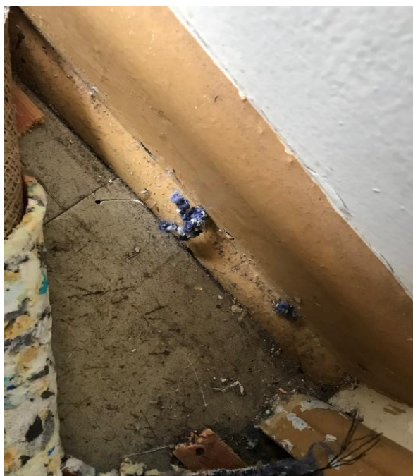
Photograph 7: B00P, R0002 - Storeroom , floor, vinyl tiles, asbestos detected by analysis.
