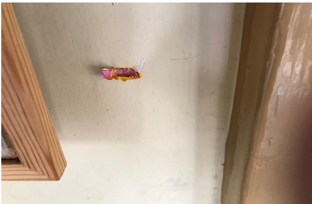
Photograph 3: B00N, exterior, throughout , undercoat to walls, white paint, positive for lead.
