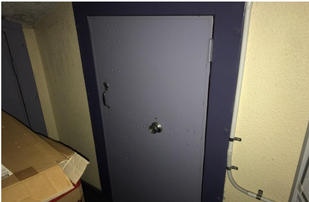
Photograph 4: B00B, R1001 - Special Programs Room, potential fire door to rear of room, internal insulation, asbestos (assumed).
