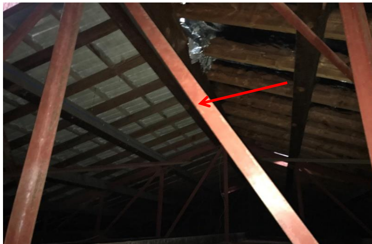
Photograph 6: B00R, interior, ceiling cavity (accessed through R0010), steel beams , red paint, positive for lead.
