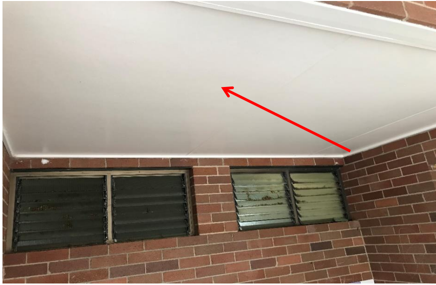
Photograph 7: B00R, R0011 - Drinking Facility , ceiling, fibre cement sheet, asbestos detected by analysis.
