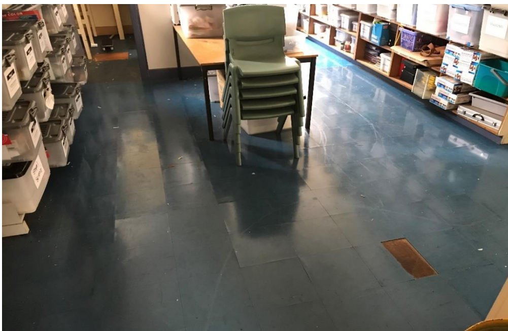
Photograph 3: B00K, R0008 - Special Movements Room, floor, vinyl tiles, asbestos detected by analysis.
