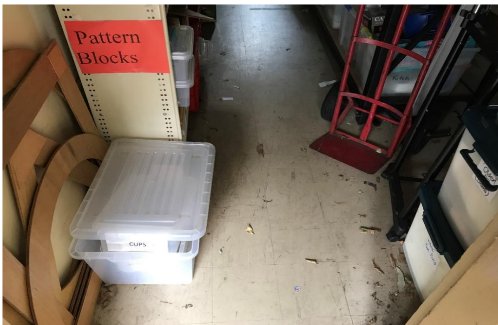
Photograph 3: B00J, R0001, floor, vinyl tiles, asbestos detected by analysis.
