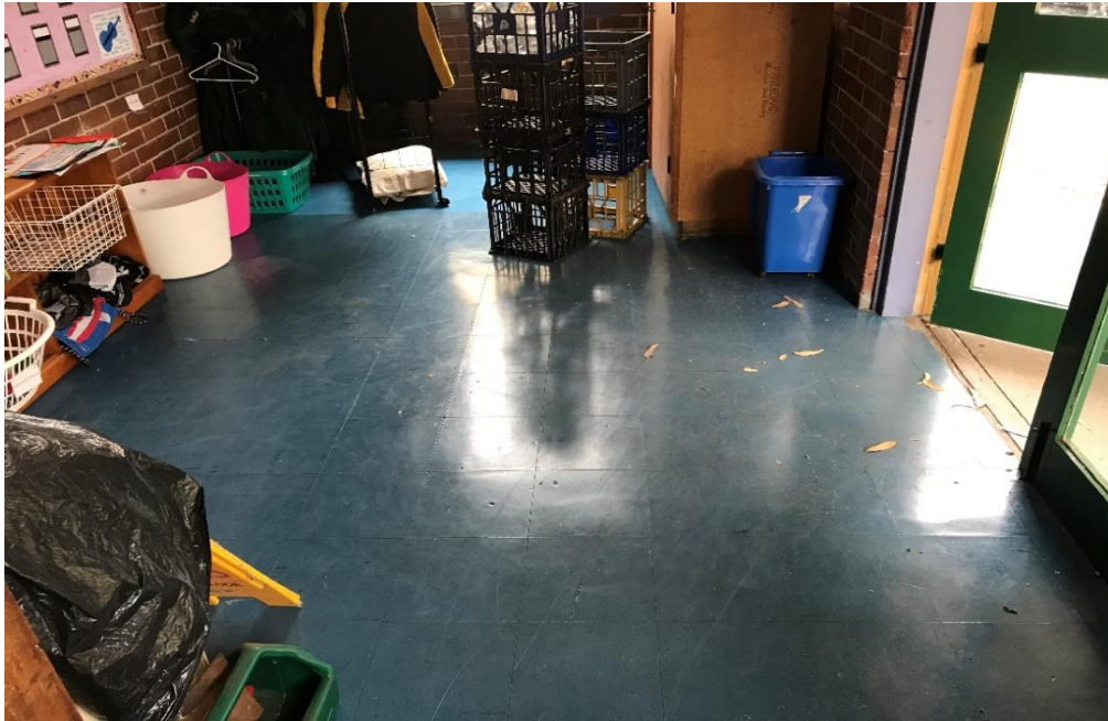
Photograph 1: B00K, R0005 - Craft Store, floor, vinyl tiles, asbestos detected by analysis.
