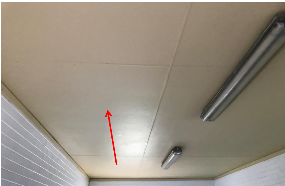
Photograph 3: B00R, R0009 - Girls Toilet , ceiling, fibre cement sheet, asbestos detected by analysis.
