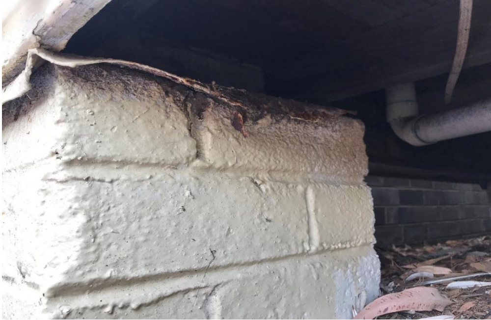
Photograph 1: B00N, exterior, subfloor, packing to piers beneath metal ant cap, fibre cement fragments, asbestos detected by analysis.
