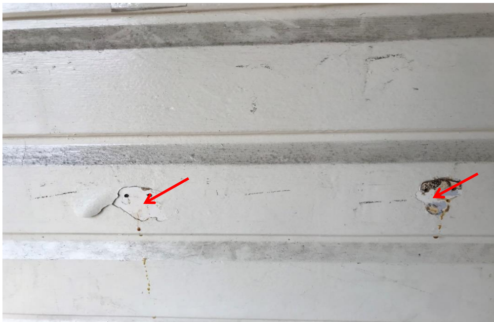
Photograph 2: B00S, exterior, throughout, walls, undercoat , white paint , positive for lead.
