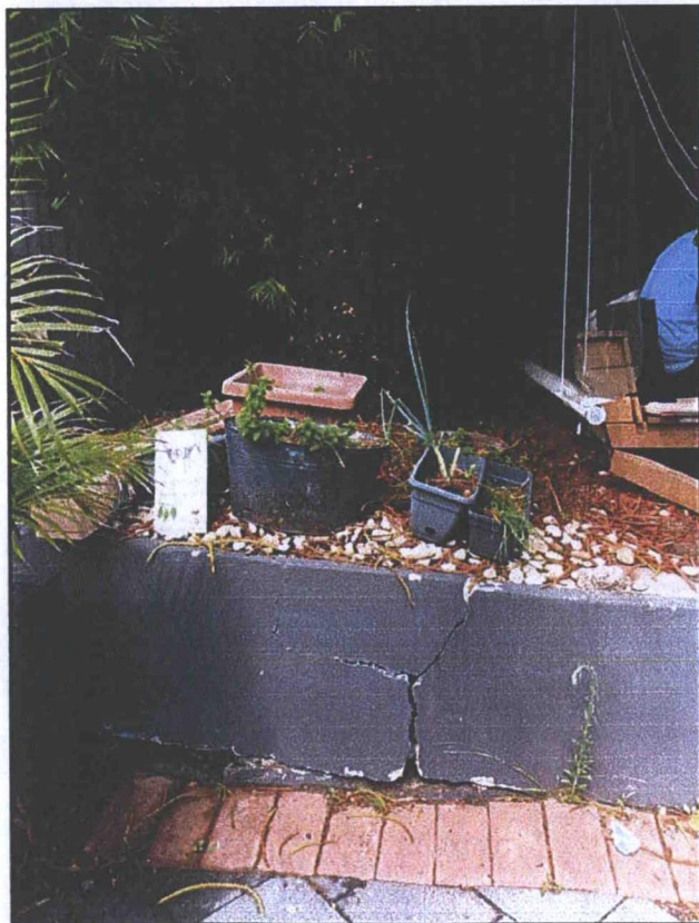
Figure 3: Damage to the retaining wall.
