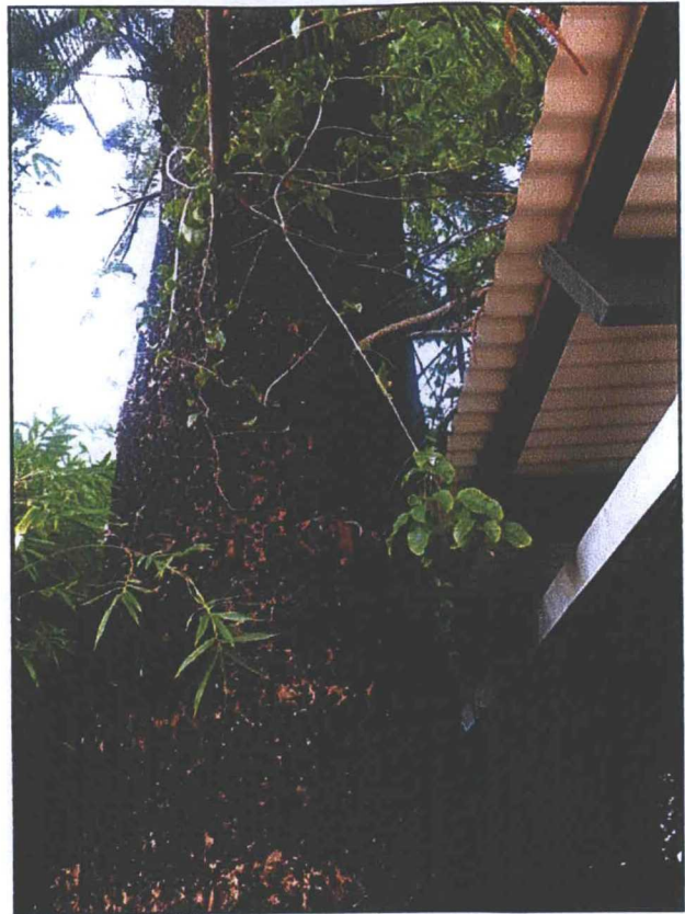
Figure 2: Trunk of the tree rubbing against roof.
