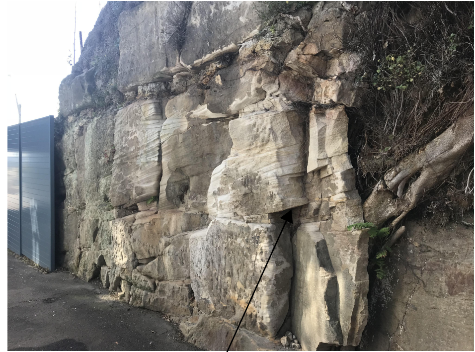
Vertical jointing observed in the cliff face
