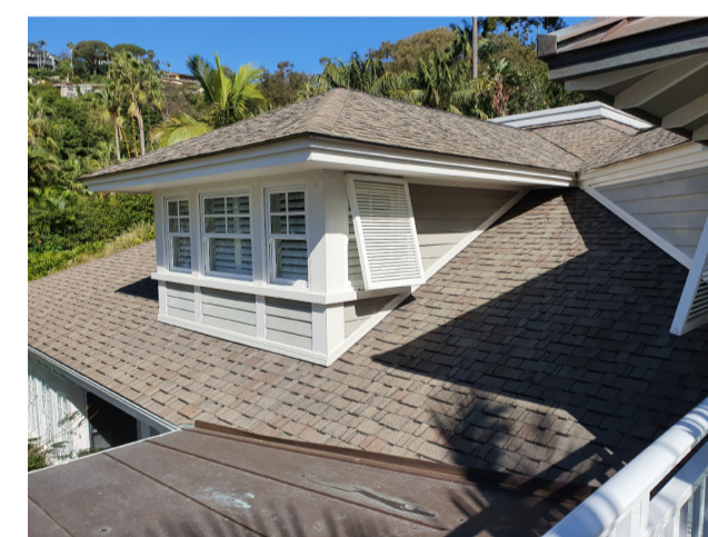
4. Shingles roof American Shingles To match existing roof Profile - Independence Colour - Weathered Wood
