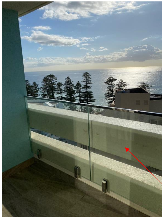
Photograph of an existing balcony and proposed balustrade – note the upper concrete component will be removed as it is non-compliant with the BCA for balustrades. The proposal is to replace as per the example above (glass balustrade)
