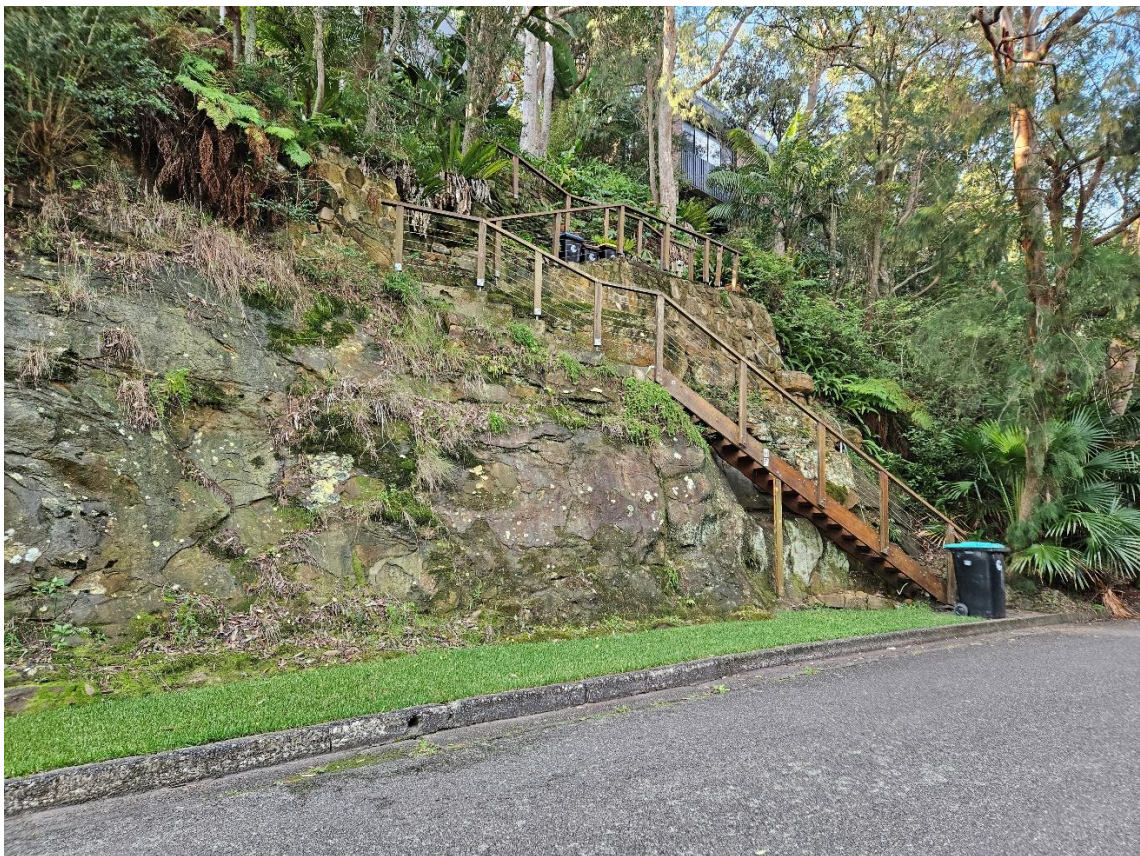
ADJOINING PROPERTY WITH AN EXTERNAL TIMBER STAIR LOCATED ON COUNCIL LAND
