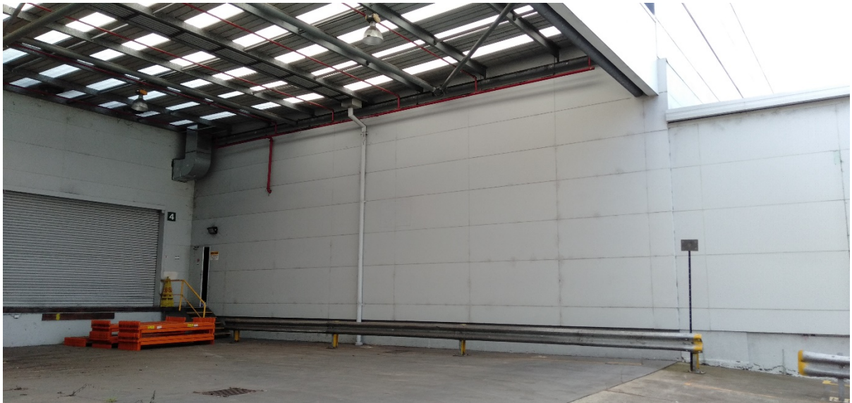
Photo 3: Loading dock at level 1 of the existing 5-storey Office and Warehouse building
