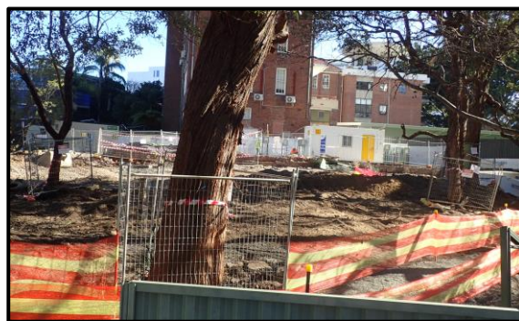
Image 2: Poor tree protection fencing not complying with AS 4970-2009. Image Paxton
