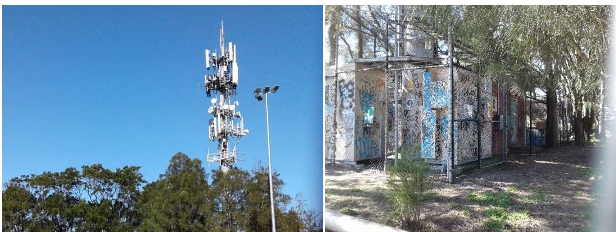
Council warn of risk that proposed tower will come to resemble similar telco facilities elsewhere on Northern Beaches. (Plateau Park, Collaroy Plateau.)
