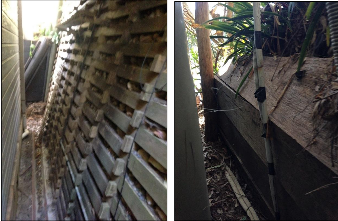
Photograph 6 and 7: Crib retaining wall below rear of existing residence (6) and timber retaining wall supporting the property to the east.
