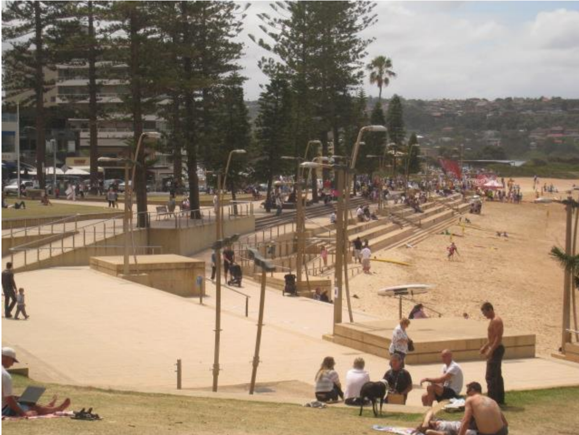
Figure 3-3 Example of colouring coastal protection works to match beach sand colour - Dee Why Beach Seawall
