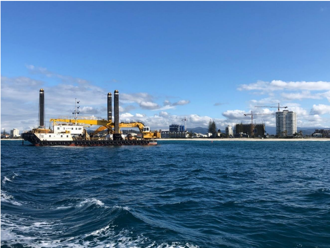
Figure 4-3 Close up view of the backhoe dredger (BHD) used in construction of the Palm Beach artificial reef
