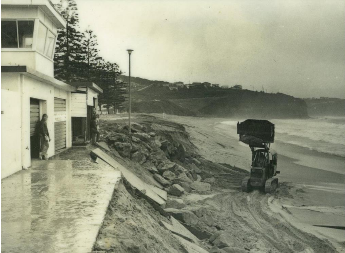
Figure 2-1 Rock protection being placed seaward of the SLSC building on 28 May 1974 (source: HCE, 2021a)
