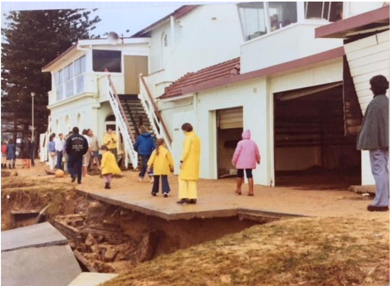
Figure 2-6 Damage to Newport SLSC from the coastal storm in May 1974 (source: HCE [2021a]).
