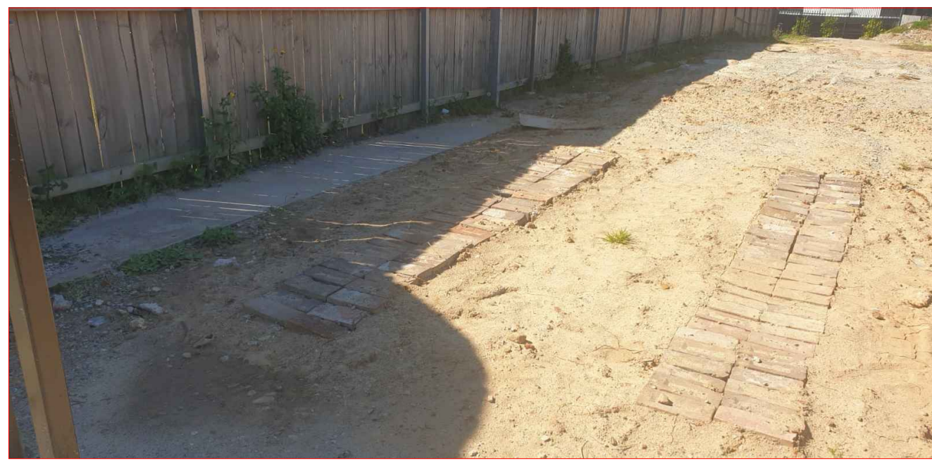
EXISTING CONCRETE TO BE REMOVED AND SEND TO RECYCLING FACILITY. BRICKS TO BE REUSED IN CONSTRUCTION OF OSD & PITS. CAN ALSO BE USED IN SET OUT DURING INITIAL WORK.
