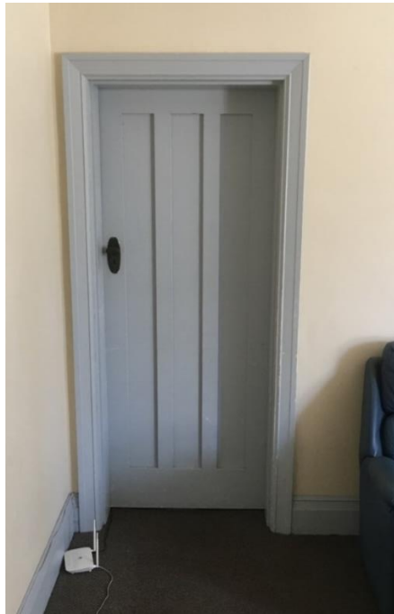
Figure 27: First floor south unit with original door detailing. Note splayed skirting on left side of the photograph.
