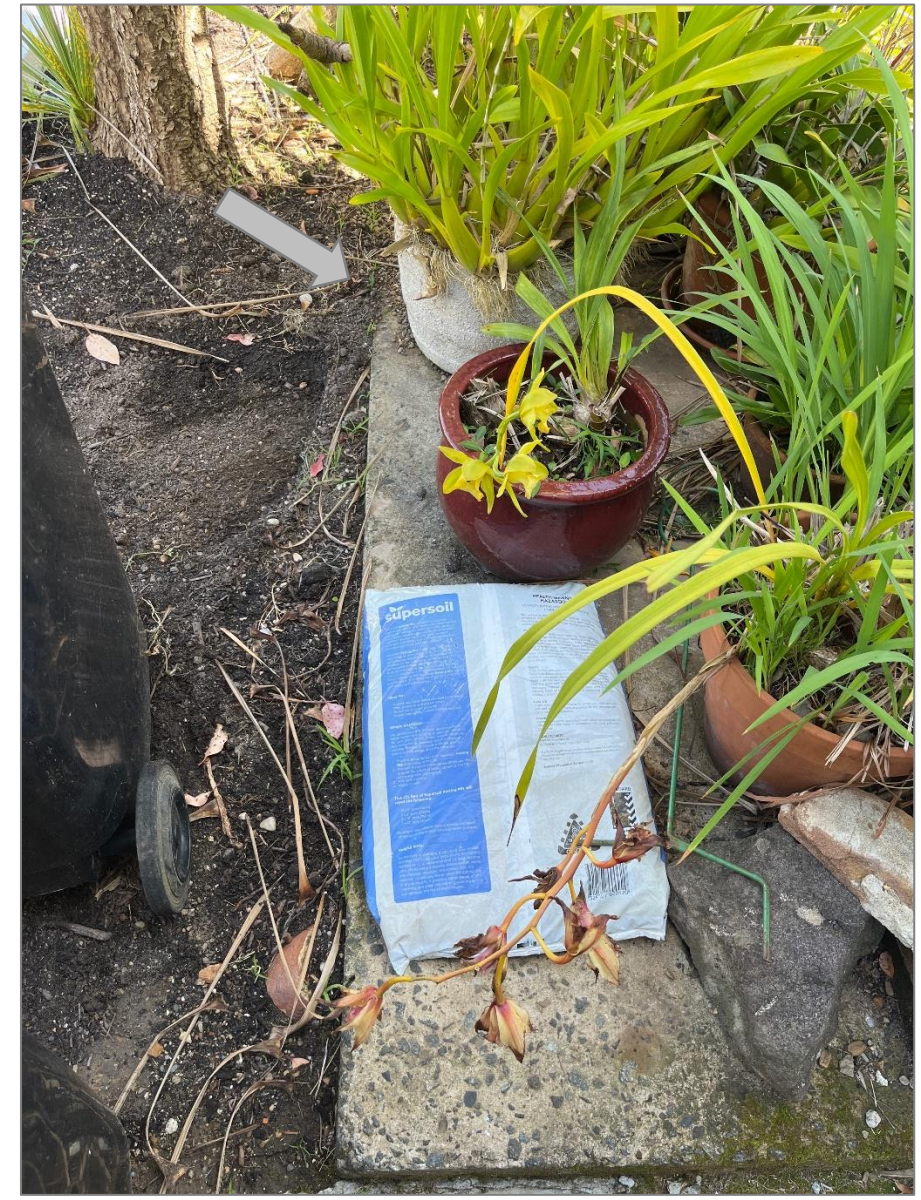
Plate 4 – Arrow notes concrete lid/slab at base of stem of Tree 5.
