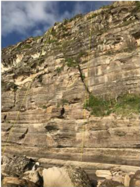
Figure 5: View of cliff face and rock platform at subject property on 7 April 2018, looking SW, with approximate lot boundary depicted
