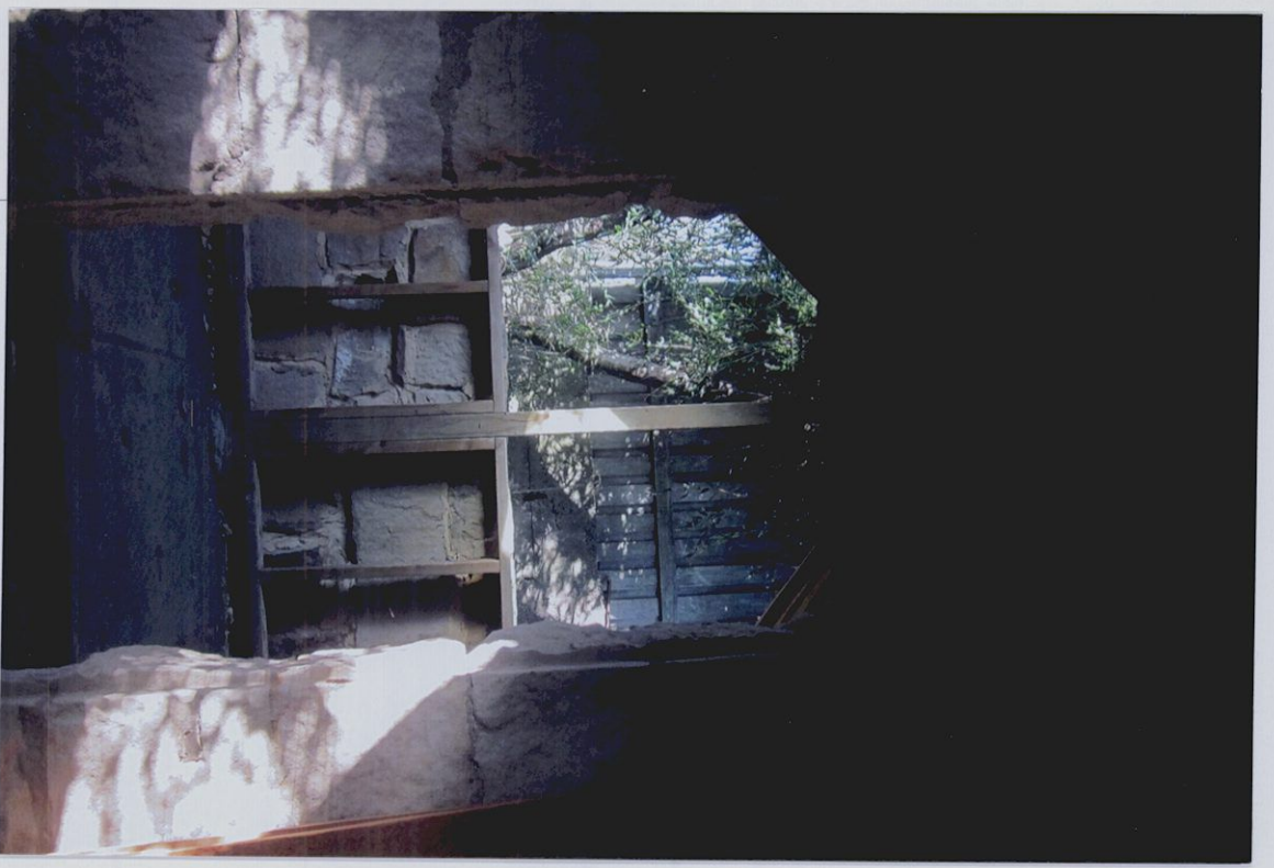
View into interior of room showing the retaining wall of adjoining property (1.8 metres distant).
