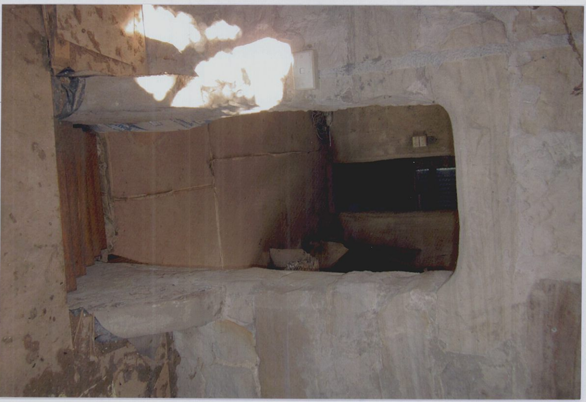
View from main bedroom to living area below. Note restricted head room and access down 5 steps.
