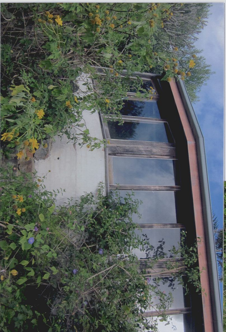
View from the North of the sunroom showing casement windows (not original)
