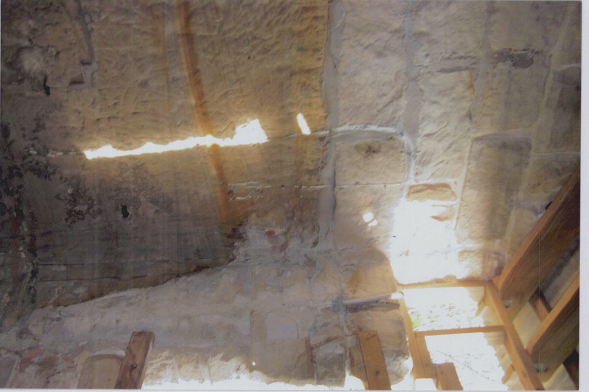
South wall of main living room showing exposed rock face to ground level with stone coursing above in designated bathroom/laundry room.
