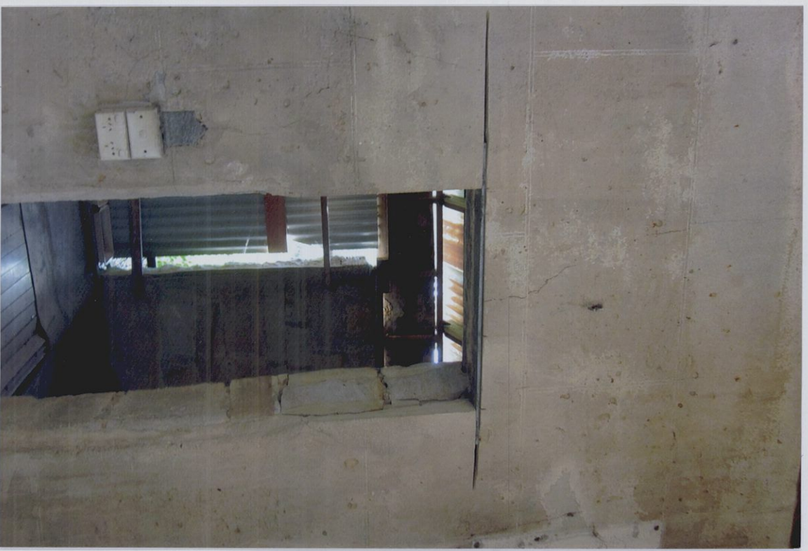
Looking into main living room. Note narrow width of doorway. (700mm). This doorway was lower, but has been heightened by a previous owner.
