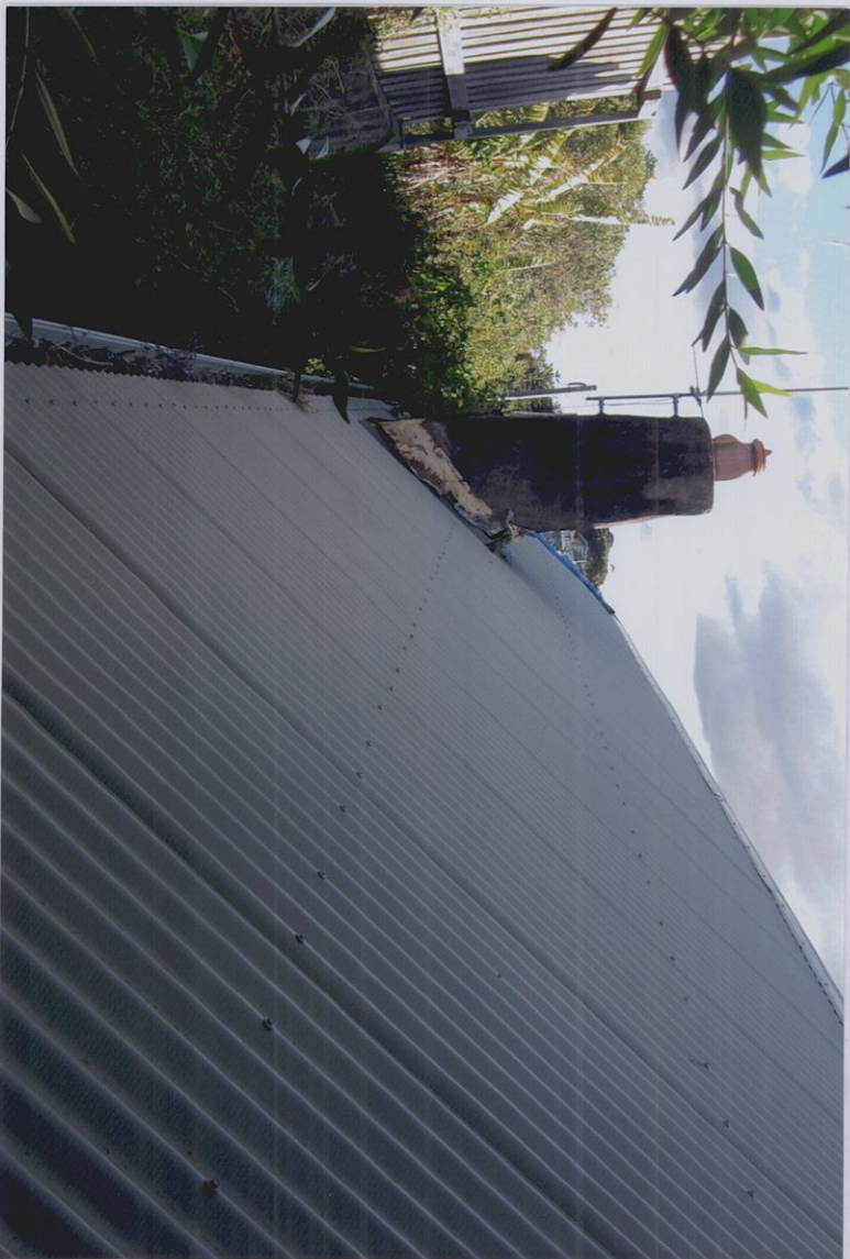
The east end of the cottage is hard up against the retaining wall of the property next door. This view shows the main roof line and rear gable.
