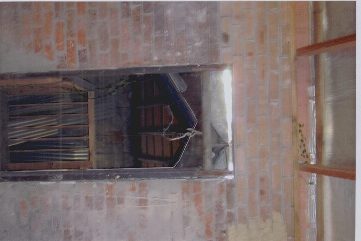
Looking into the so called "Dungeon" room showing landing and railing to staircase into this
