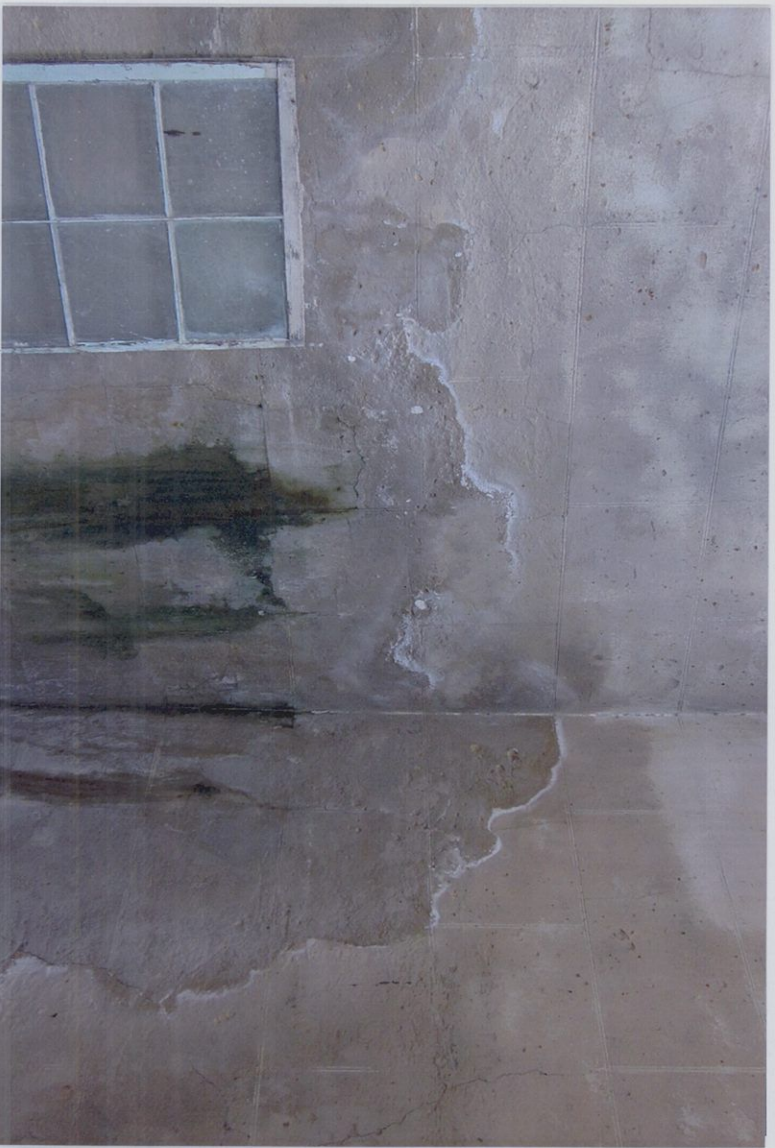
The South wall is below ground level up to a level of 2.1 metres. Detail shows water penetration through stucco/render.
