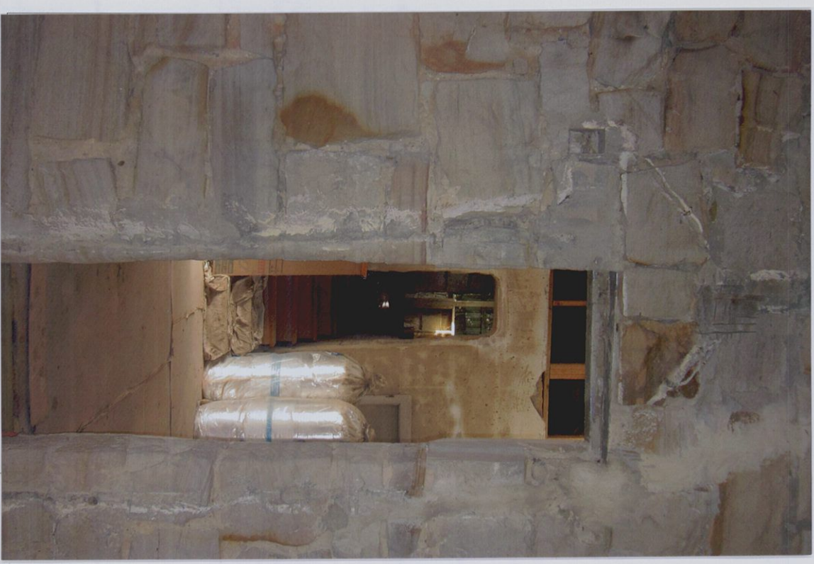
Rough nature of stonework in main living room. This is looking back
