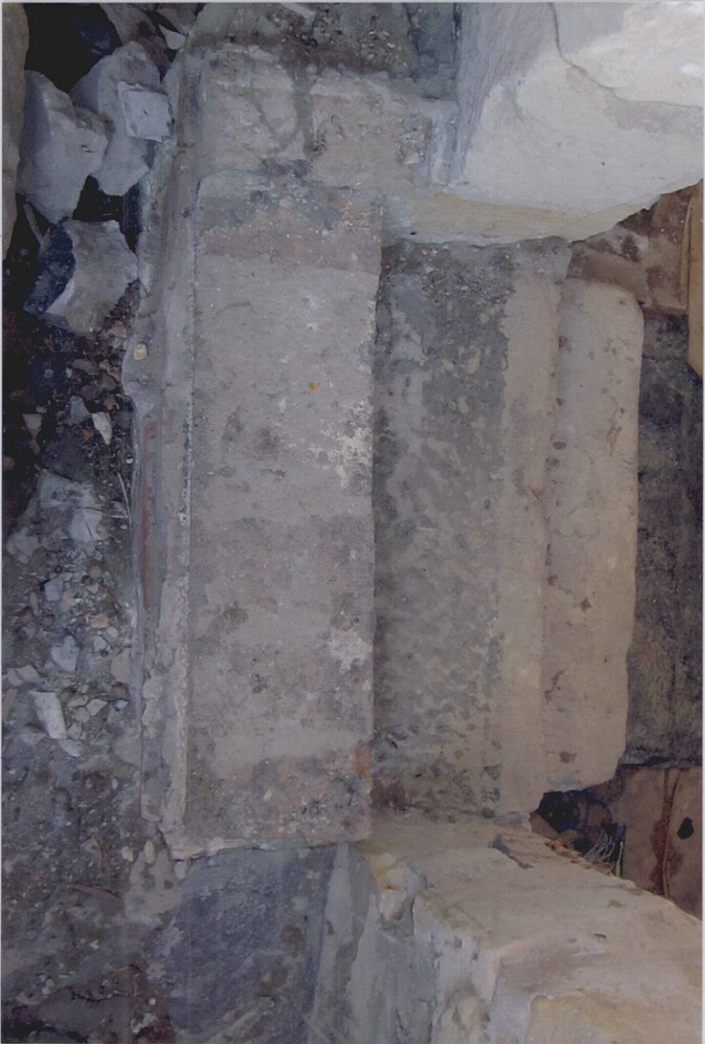
Entrance to ensuite showing original steps. A further level has been added to the floor making an additional step and restricting head room.
